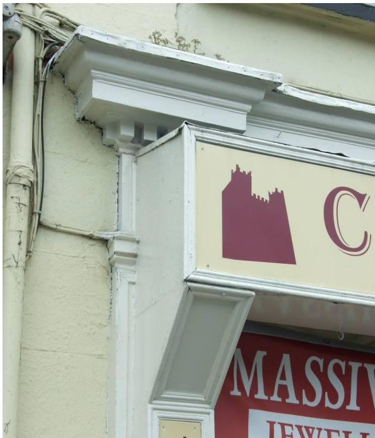
Fig. 127: Inappropriate alterations obscuring a decorative shopfront
