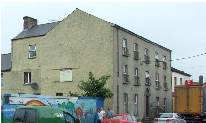
Fig. 105: Loss of chimneys upsets the proportions of this Georgian house
