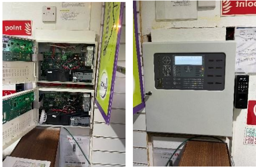
The old & new Fire Alarm Panels at Drogheda Leisure Centre
