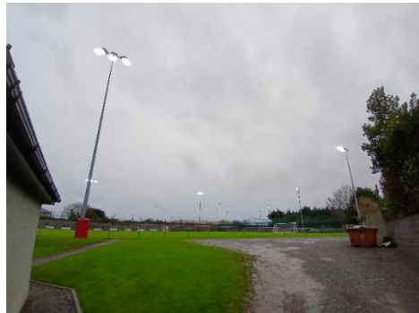
New LED lighting at Drogheda Town F.C
