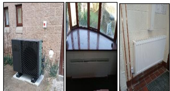
Photos showing windows Improvements, New Solar PV Inverter, New Heat Pump, New Radiators at Carlingford Fire Station
