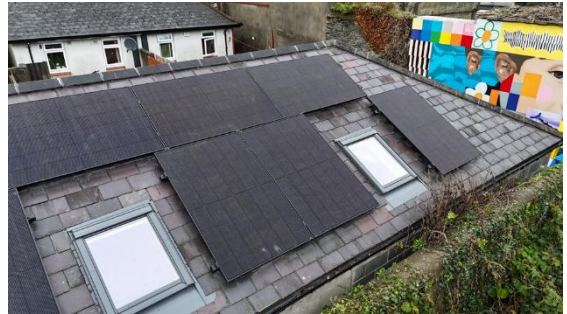
The new solar PV installation at Dundalk Outcomers
