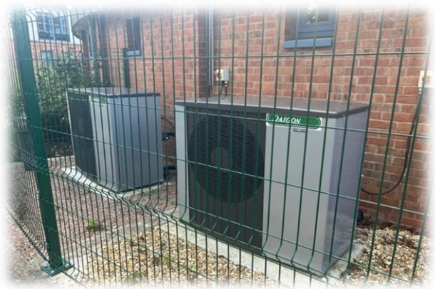
Photo 3: Air Source New Heat Pump at County Hall
