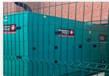
Photo 4: New Generator at County Hall
