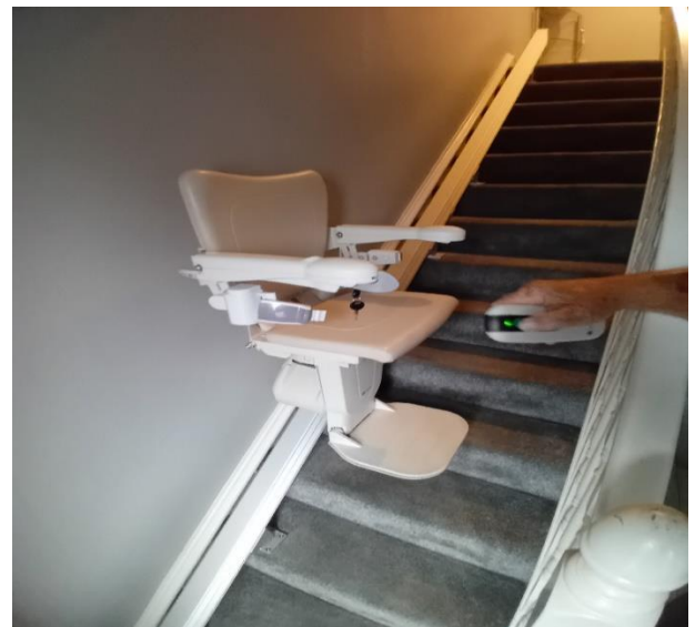
Stairlift installed in Dundalk in October, funded by a Housing Grant for Disabled Persons
