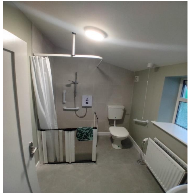
Bathroom Adaptation completed in October in Drogheda part funded by a Housing Grant for Disabled Persons
