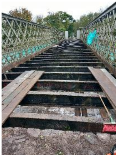
Obelisk Bridge Concrete Deck fully removed with protection sheeting laid out underneath on scaffolding platform
