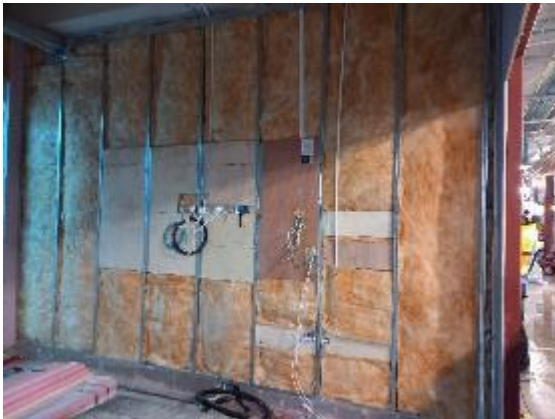
Block N: New Link Building sound insulation, grounds for AV and first fix wiring in Meeting Room
