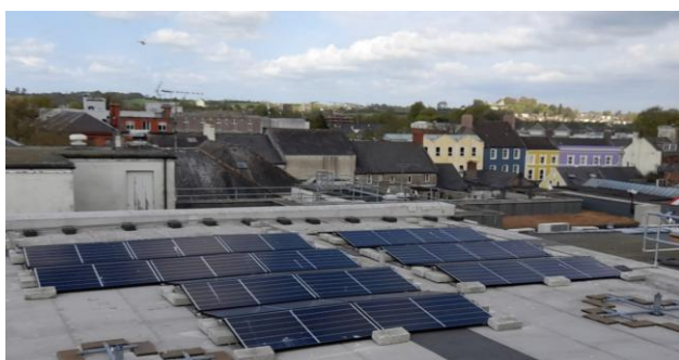
Photo 1: PV panels on Dundalk Town Hall
