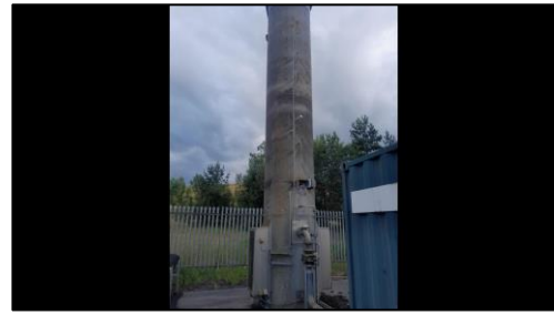
Photos: Flare and instrumentation at Whiteriver Landfill.
