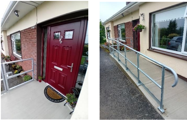
Ramp and front door completed in Dundalk, with funding provided with a MAG
