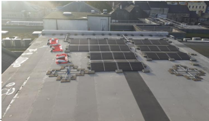
New 11KW Solar PV Electricity Generator at Dundalk Town Hall
