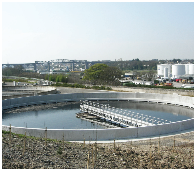
Drogheda Waste Water Plant
