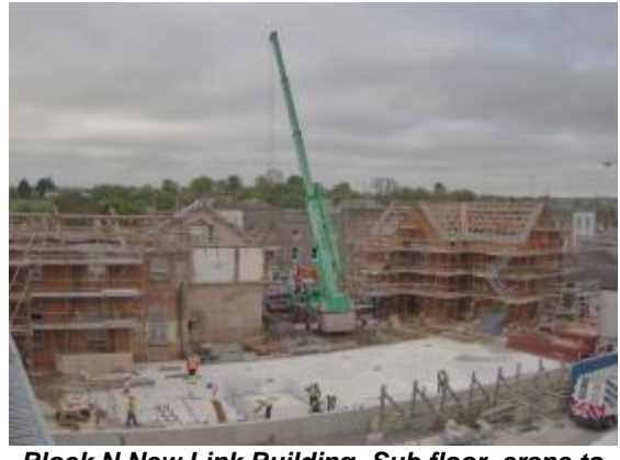
Block N New Link Building- Sub floor, crane to commence erecting steel frame
