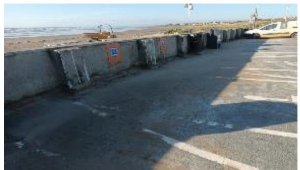
Sand Cleared at Clogherhead Car park
