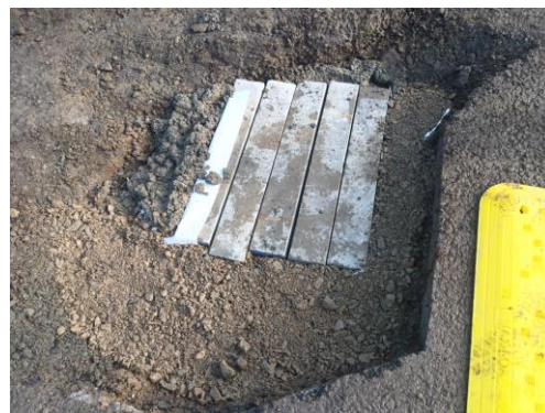
Culvert Collapse in Tinure
