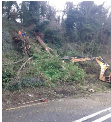
Fallen Tree N51 Drogheda Slane Road requiring emergency Road Closure
