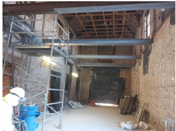
Shot blasting Fire damaged Steel Beams prior to Intumescent Paint application Block B – Council Chamber
