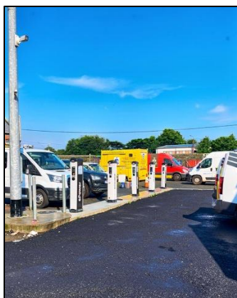
New EV Charging Equipment at Dundalk Machinery Yard
