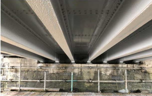
Span 4, two coats of paint have been applied and new bearing bads replaced
