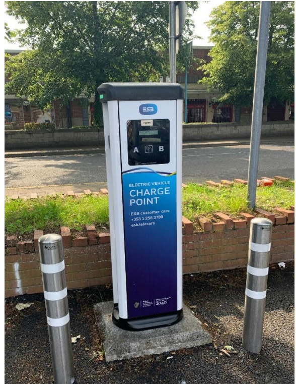
EV Charging Point
