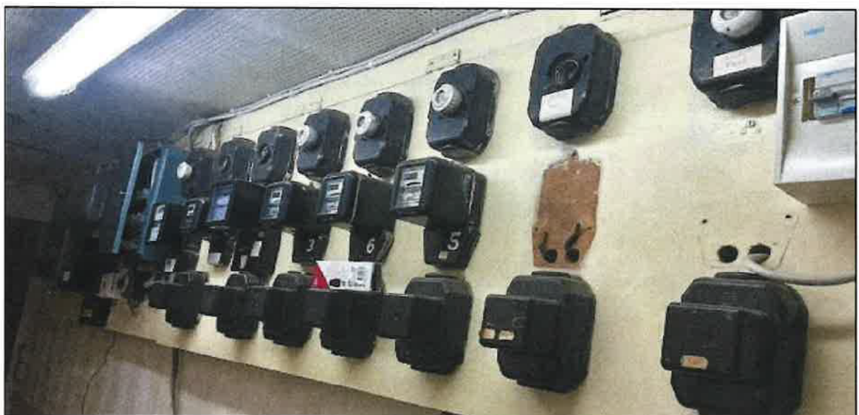
Figure 4.0 Image showing the electric meters for each apartment.
