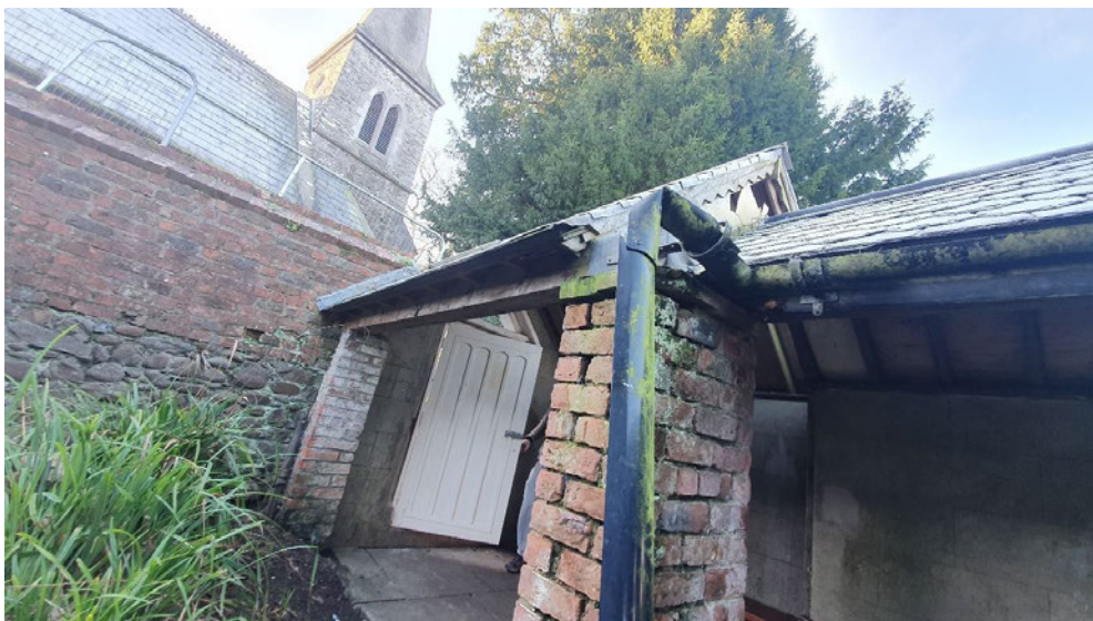
Gutter to be replaced
