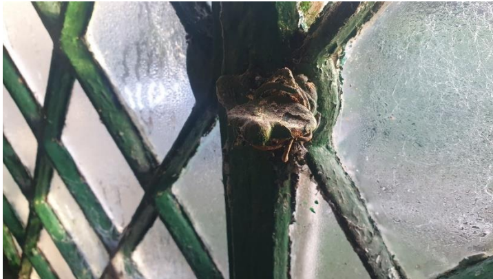
Latches not functioning on many windows.
