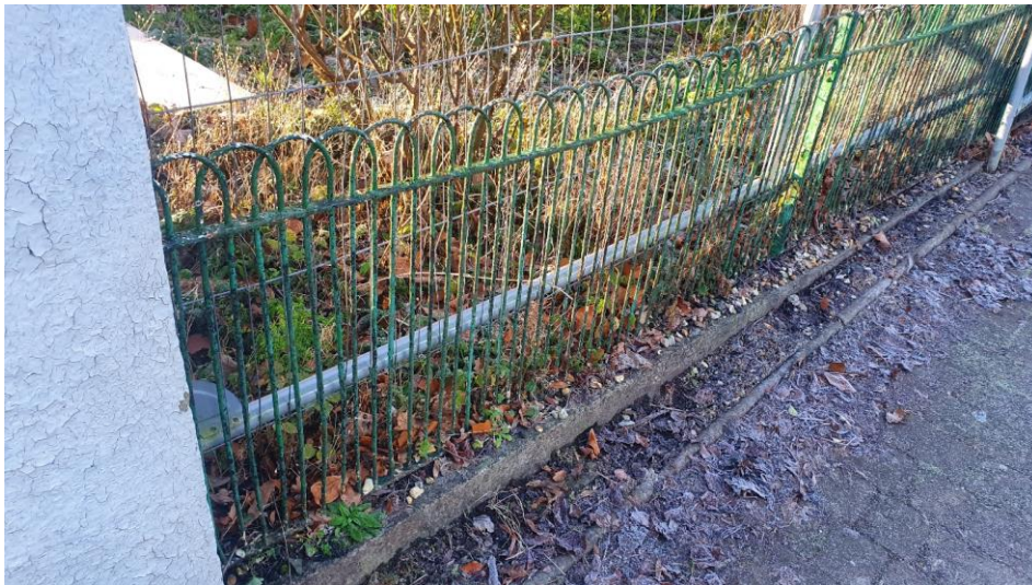
Overlapping bowtop railings
