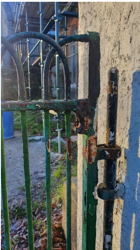
Corrosion and flaking paint.
