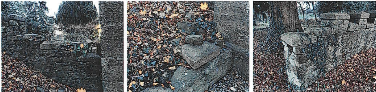
Figure 2: Views of existing stone walls at gate piers to be repaired.
