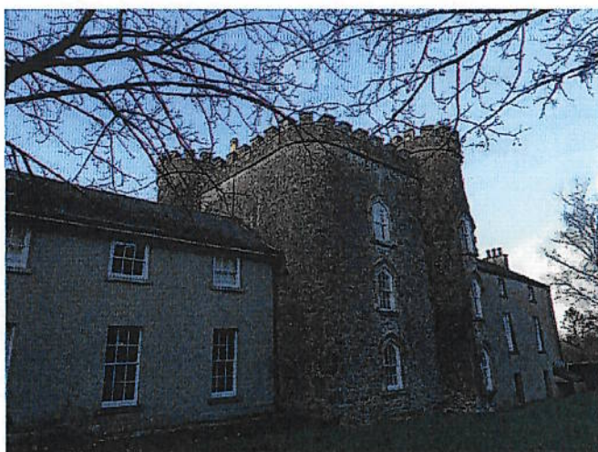
Figure 3: Views of castle tower (flat hidden roof to be repaired)
