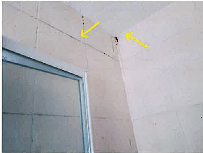
Sample of apparent mould in bathroom.
