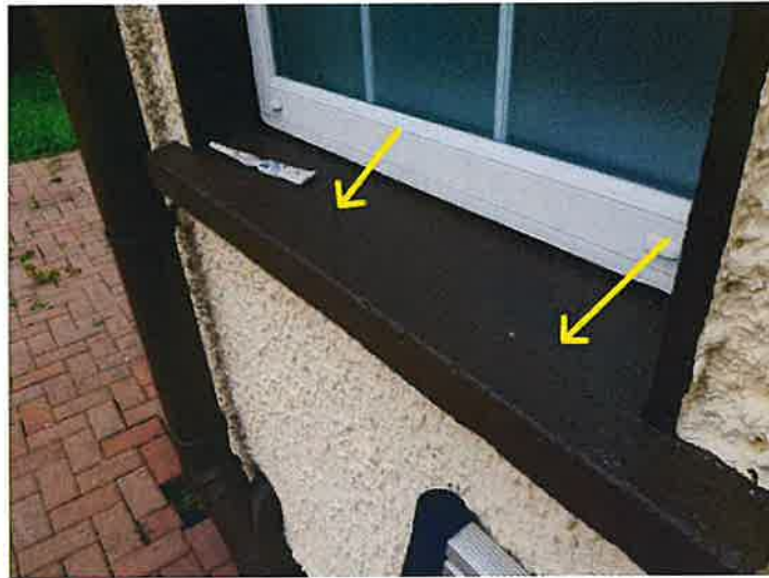
Repair cracked / damaged window sills.
