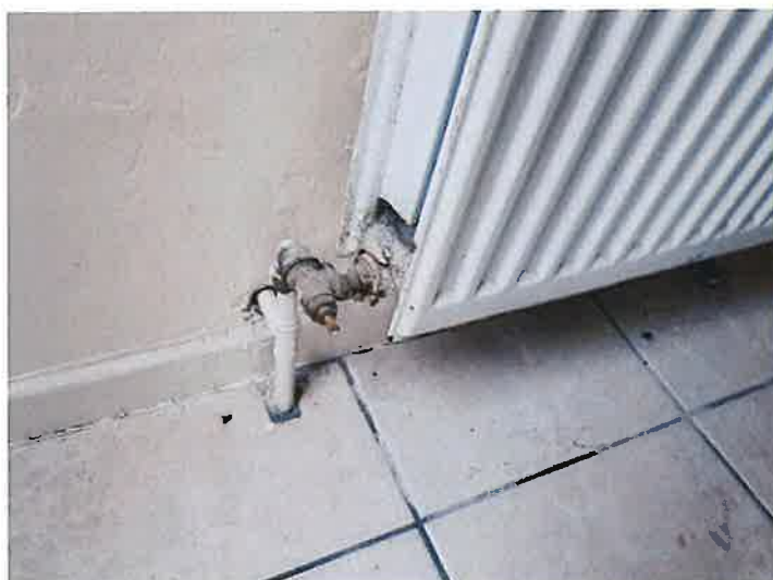
Sample of valve covers missing to radiator pipes.
