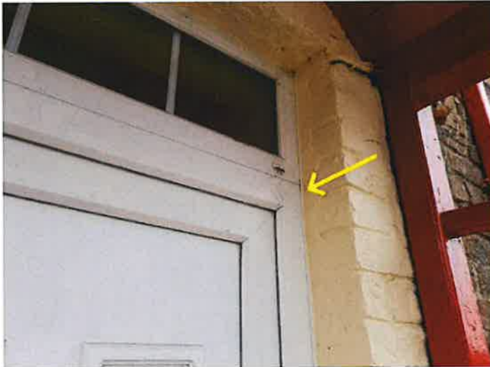
Re-seal around door frame/s.
