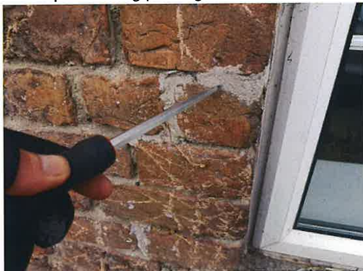
Sections of brickwork walls have been repointed with a cement based mortar, a lime based mortar should have been used.
