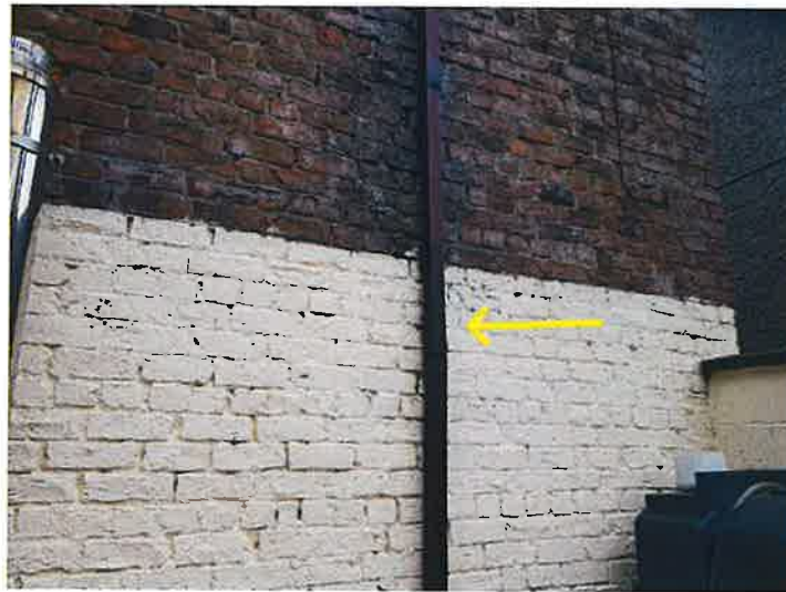
Secure loose downpipes to property.
