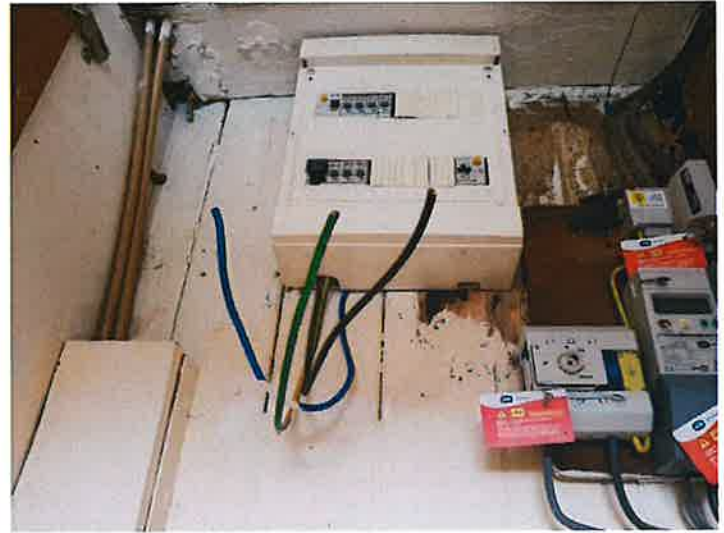
Electrical breaker panel not connected to meter.
