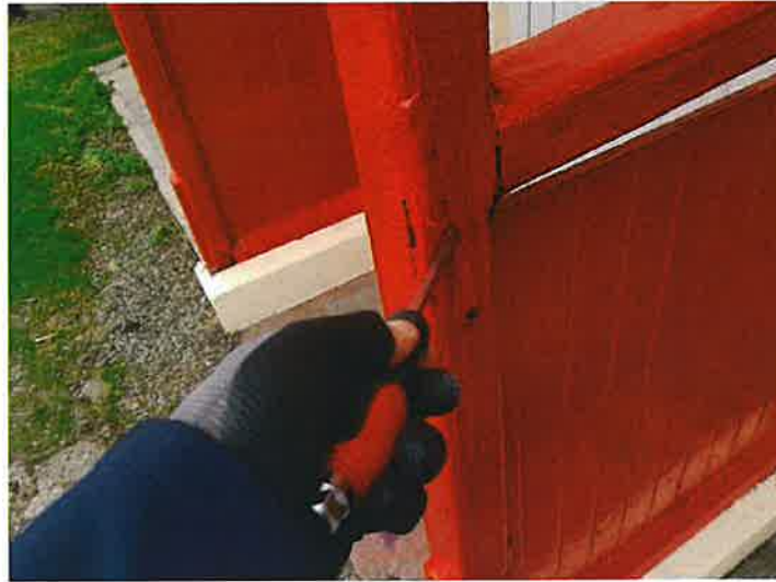
Rotten timbers supporting canopy
