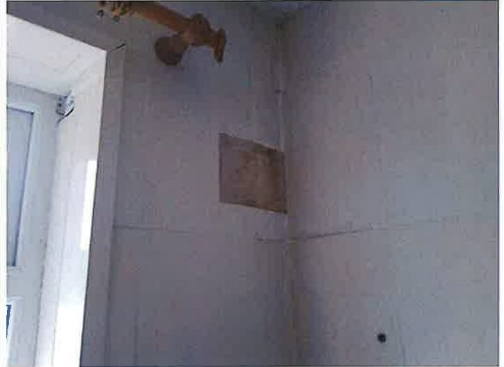
Vent opening partially blocked in bathroom.
