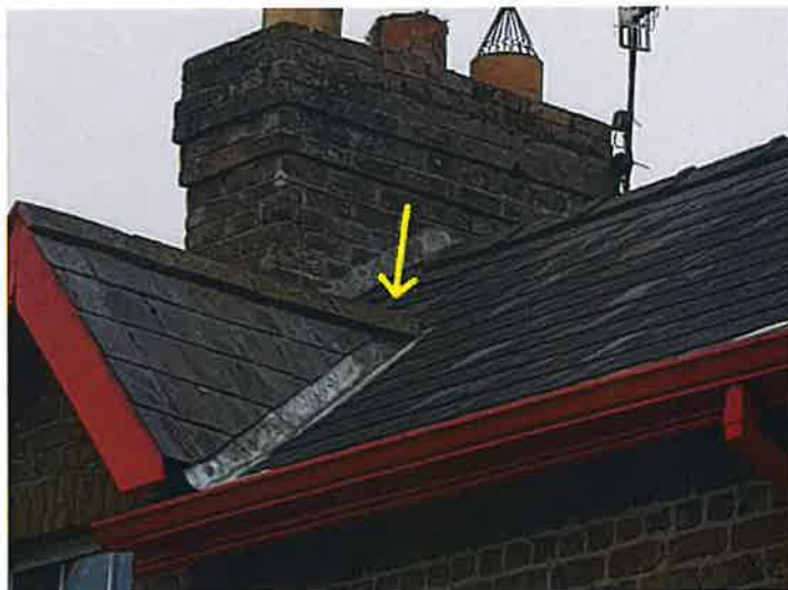
Sample of cracked / damaged roof covering.
