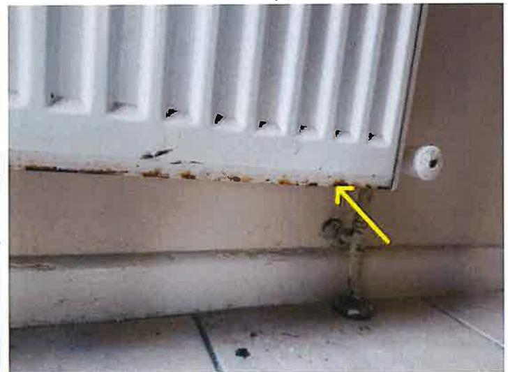
Sample of corrosion in radiator to property.
