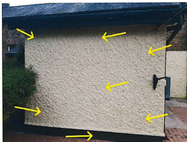
Sections of dashing (hollow sound with some cracking) not fully bonded to masonry walls, will require local repairs.
