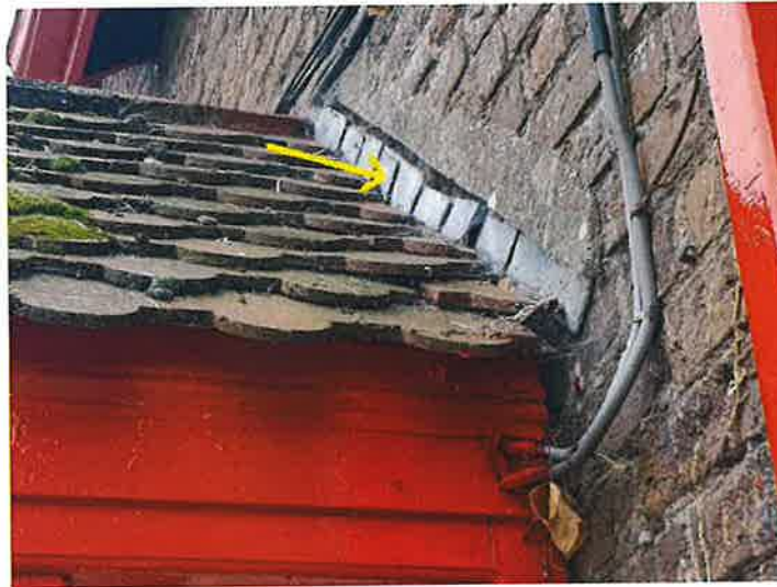
Re-secure / repair flashing to front canopy.
