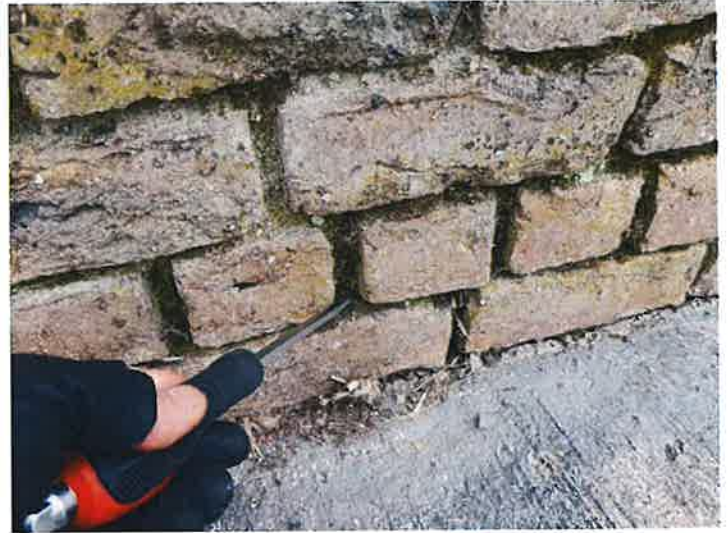
Sample of failing pointing between brickwork.
