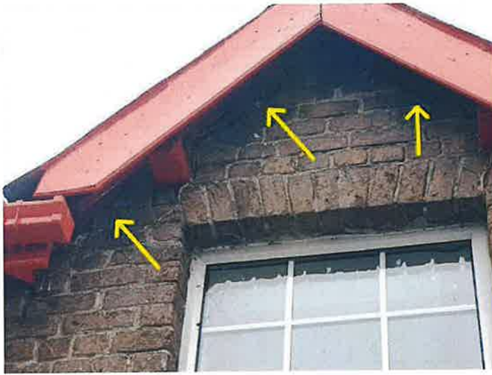
Remove vegetation and seal gaps between brickwork walls and soffits
