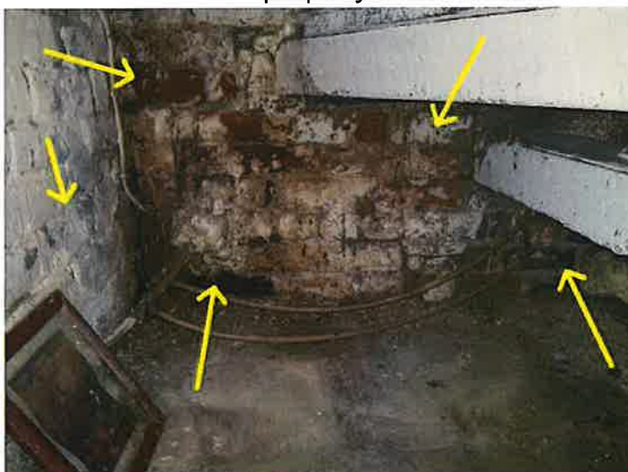
High moisture readings noted to back wall of property.
