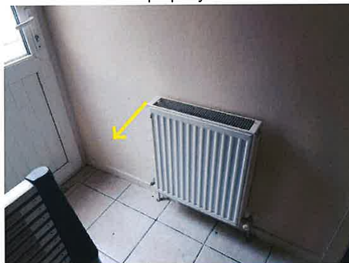
Normal moisture level reading taken at internal wall of property.
