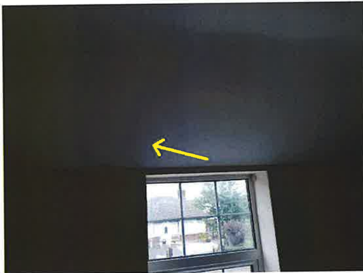
Sample of crack/s in ceilings.
