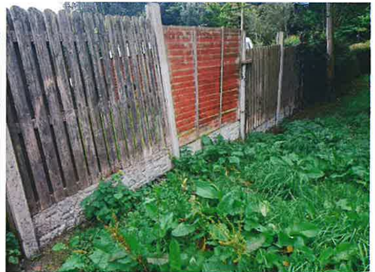
Delayed maintenance to boundary fences.
