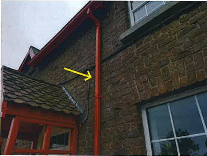
Secure loose downpipes to property.
