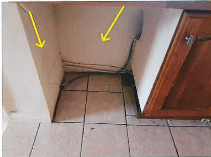
High moisture readings noted to back left wall of property.
