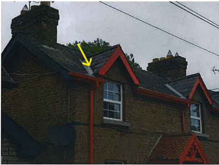
Sample of slipped roof covering.
