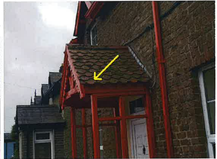
Sample of missing roof covering.
