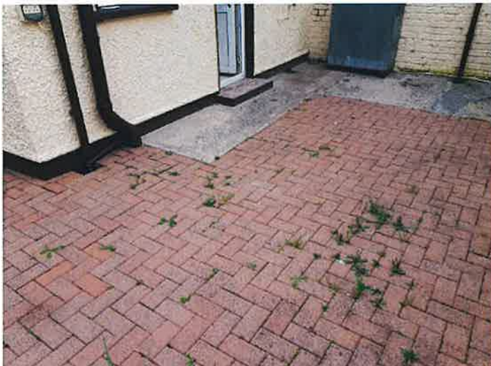
Inadequate access to drains, no visible inspection chambers.
