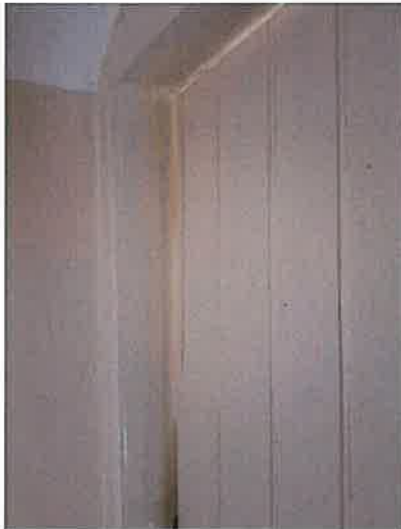
Doors to bedrooms not sitting square on door frames.
