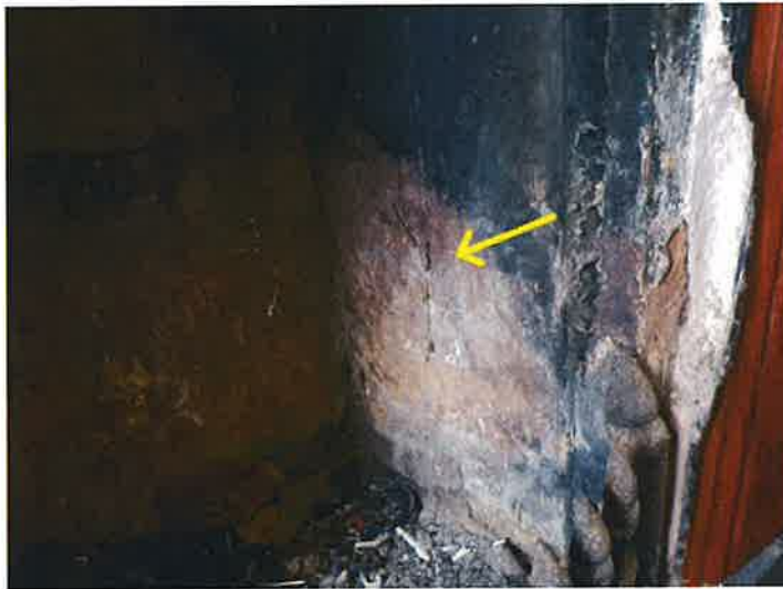
Repair damaged firebrick in fireplace.
