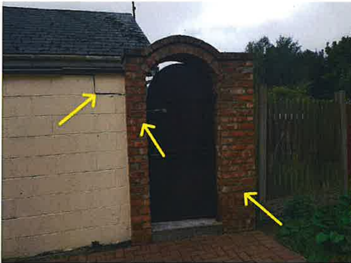
Sample of settlement in back left boundary wall/ arch.
