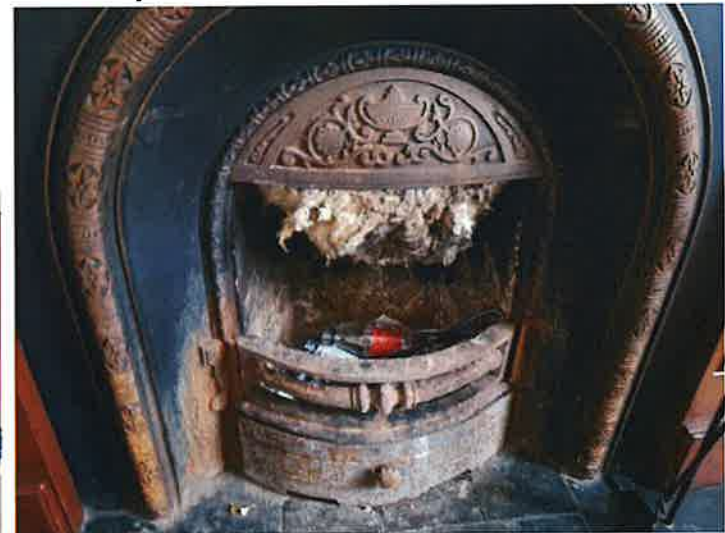
Treat rusted fireplace
