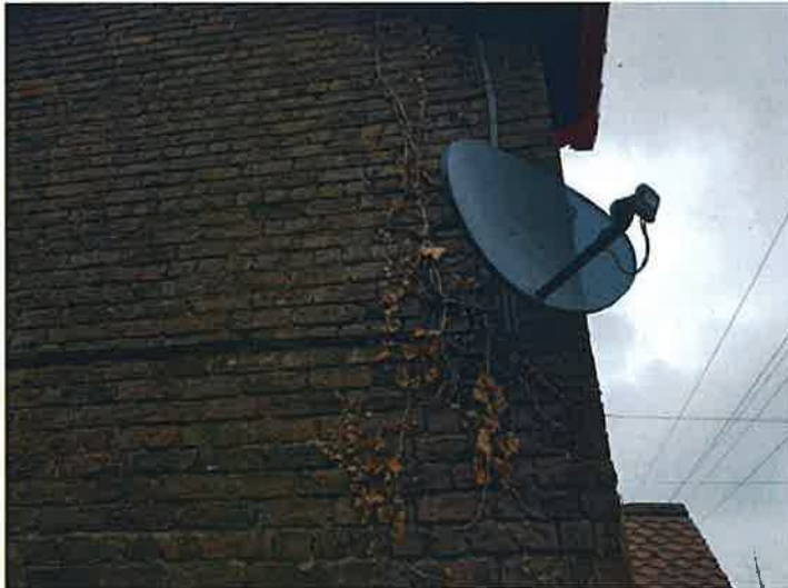
Vegetation partially restricting view to exterior wall.
