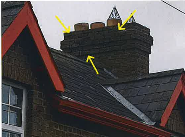
Repoint brick chimney. Brick and mortar deterioration observed; repair advised.
