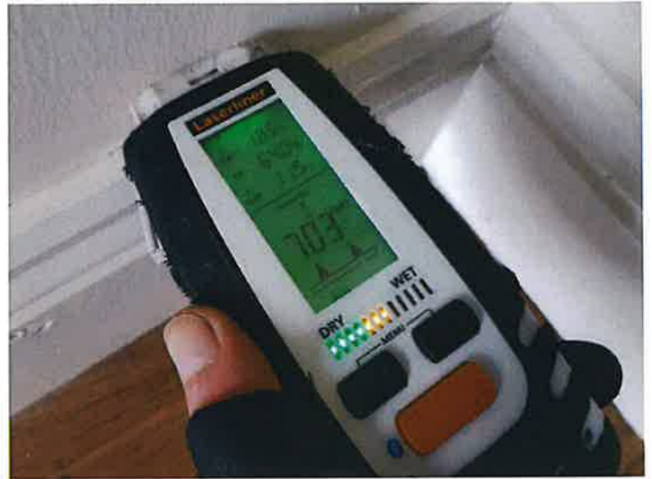
High moisture readings noted to left wall of property.
