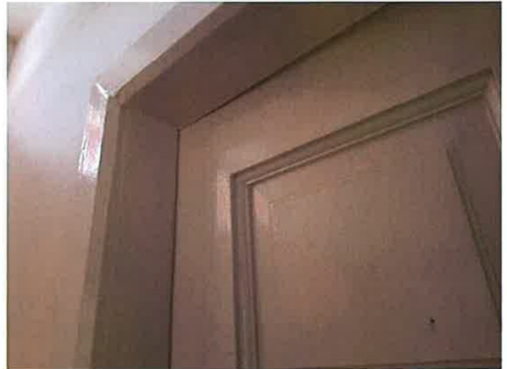
Door to left side living room catching on door frame.
