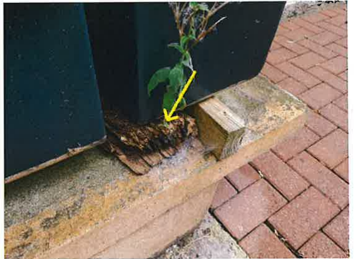
Rotten timbers supporting oil tank
