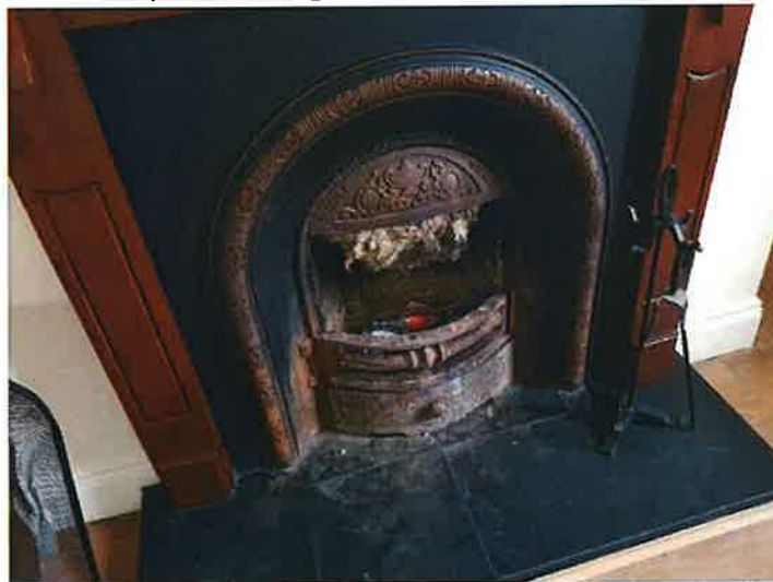
The fireplace/s would appear to be in a fair condition where visible.
