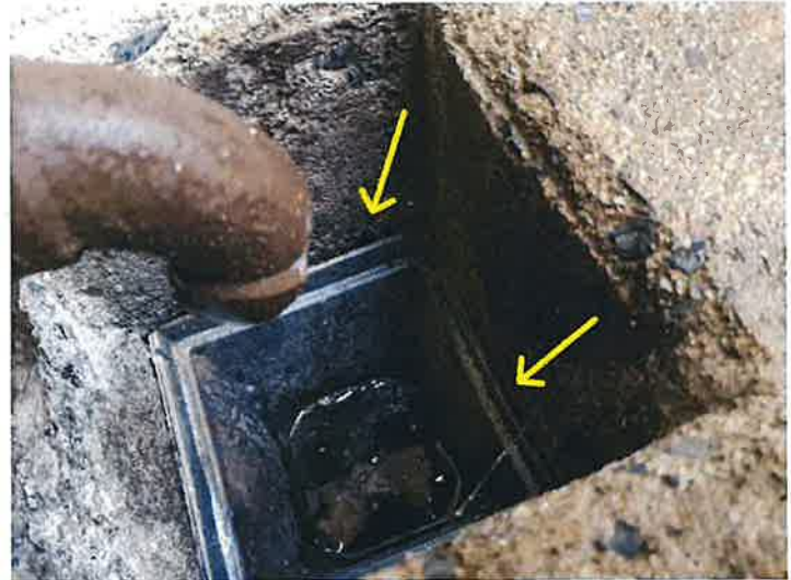
Gaps present which can allow water seep into the ground around the walls of the property. Repair.
