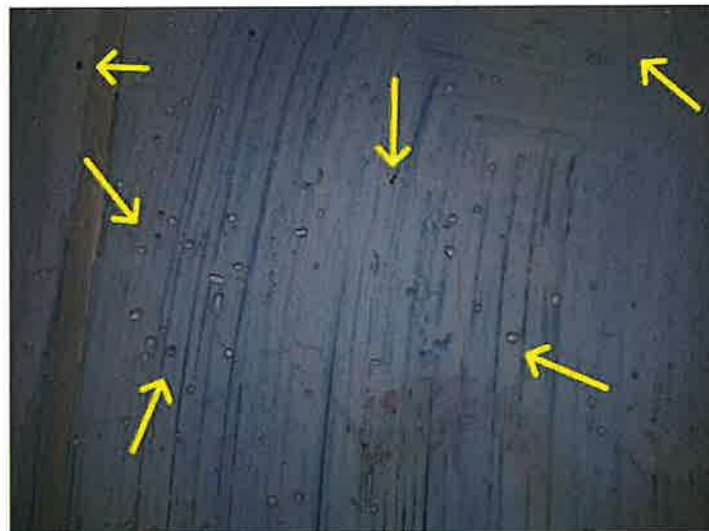
Sample of active woodworm in stairs timbers.
