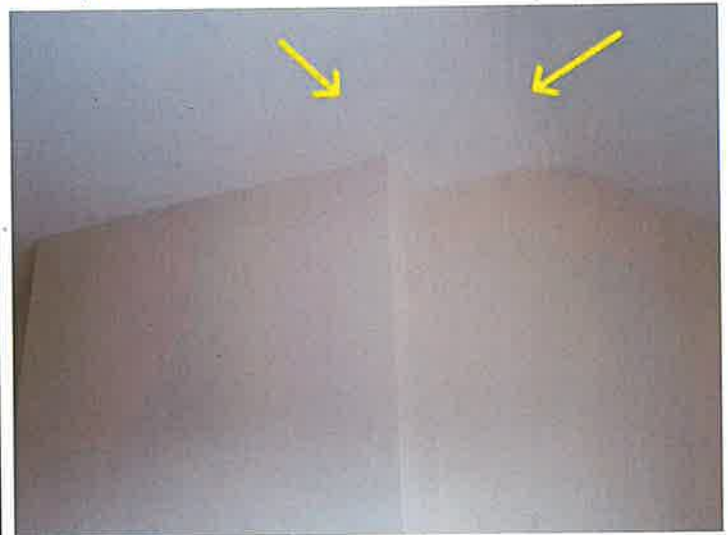
Moisture stains/ patched repairs in right bedroom ceiling adjacent to chimney. Dry at the time of inspection, further investigation / repairs required.
