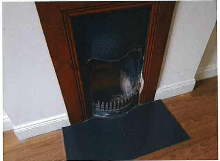
The fireplace/s would appear to be in a fair condition where visible.
