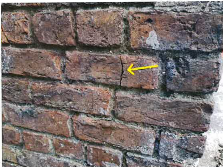
Sample of cracked brickwork in left wall.
