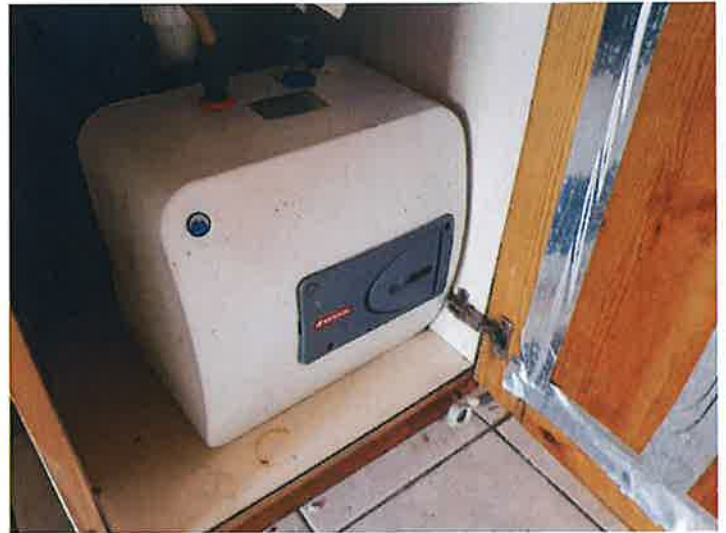
Under sink water heating unit not functioning, no power to same.
