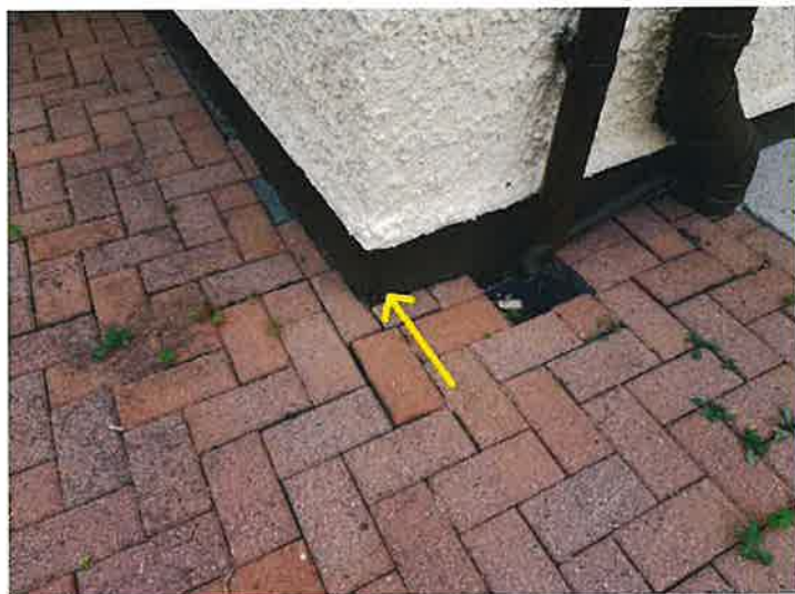
Sample of chipped render in back wall.
