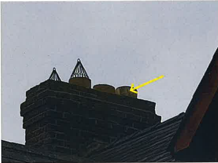
Replace / repair chimney capping / pot/s.
