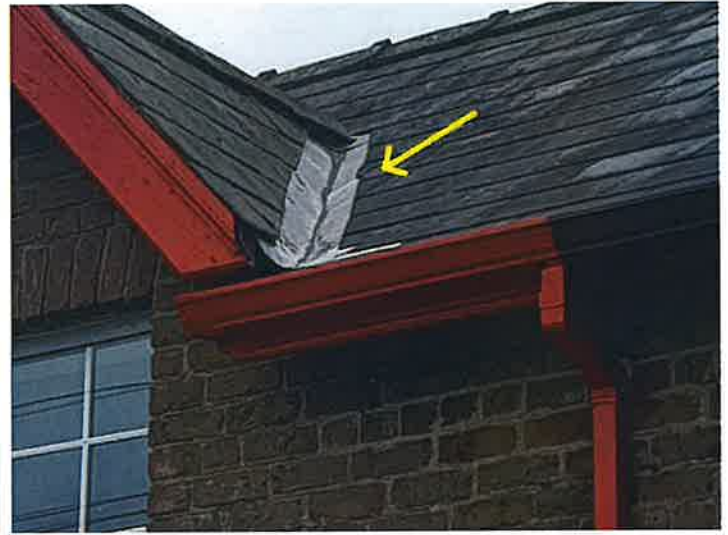
Sample of slipped roof covering.
