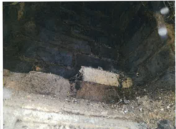
Chimney flue, should be cleaned out before use.
