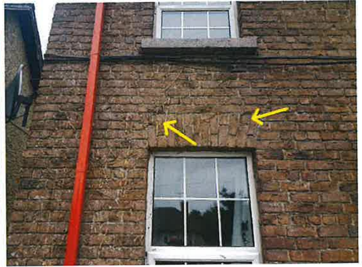
Sample of crack/s in front wall.
