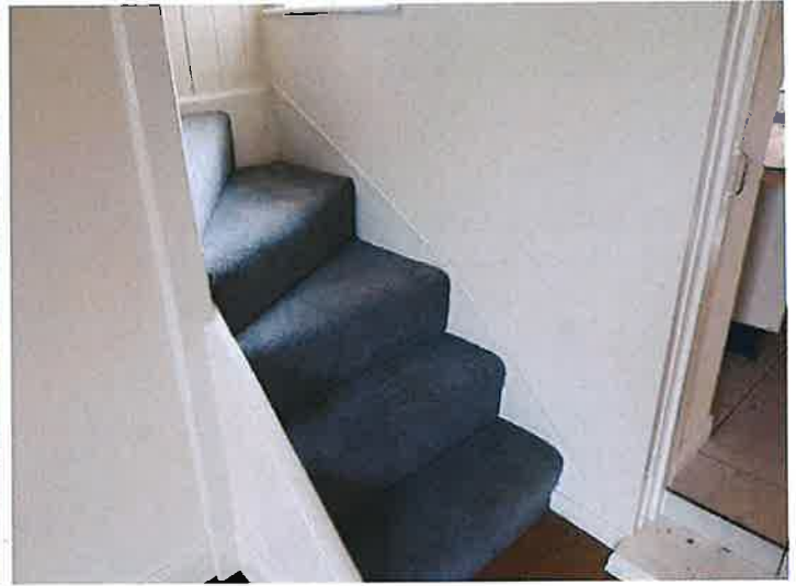
No hand rail fitted to bottom section of stairs.
