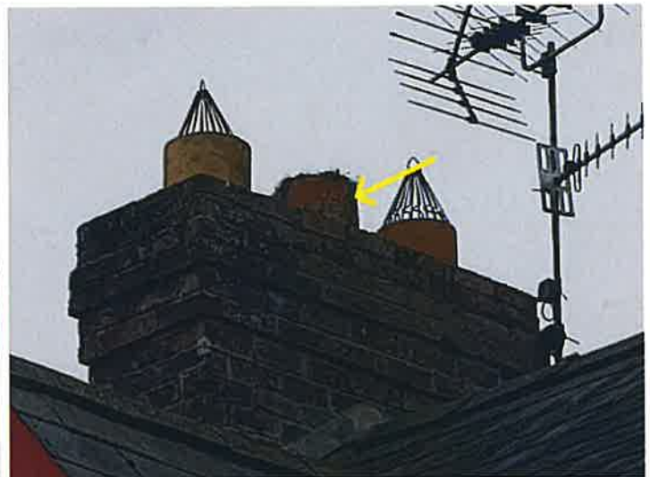
Replace / repair chimney capping / pot/s.
