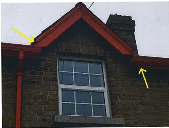
Sample of rotting sections of timber fascia and soffits.
