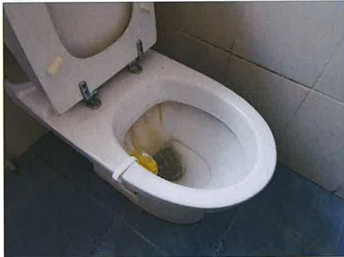
Adjustments required to toilet, running constant after flush.
