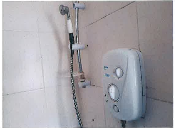
Electric shower not operating at the time of inspection. No power.
