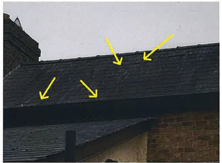
Sample of slipped/ lifted roof covering.
