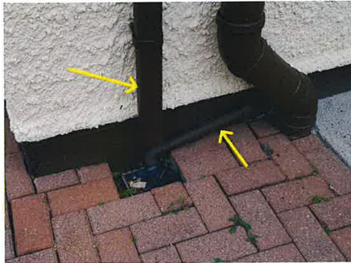
Foul and rain water discharging into same drain.
