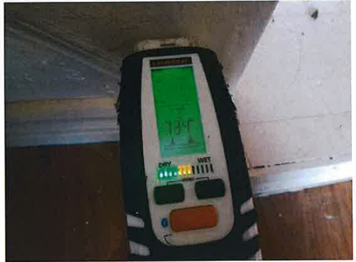
High moisture readings noted to internal wall of property.
