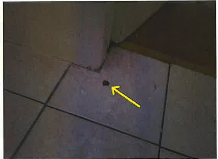
Sample of floor tiles damaged in hallway.
