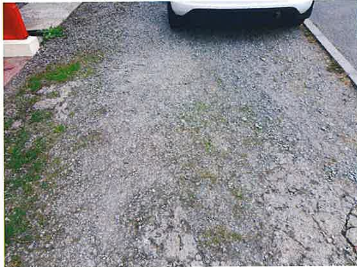
Delayed maintenance to driveway.
