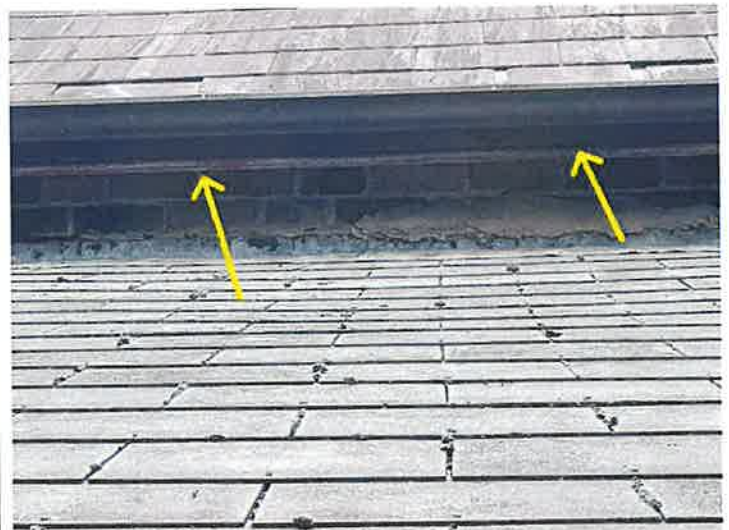
Delayed maintenance to fascia and soffits.
