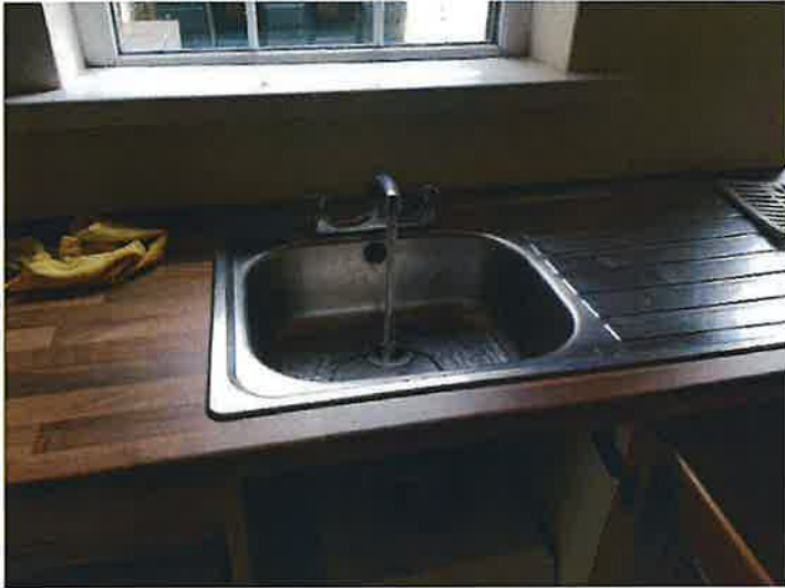
Sample of tap/s operating at the time of inspection.
