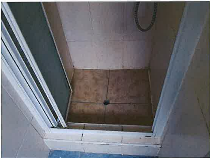
Re-seal around shower base/ screen.
