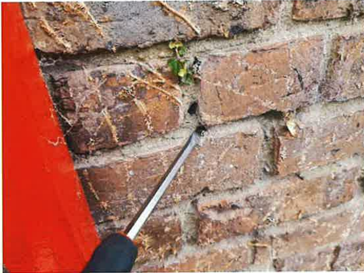
Sample of failing pointing between brickwork.
