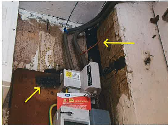
Charred timber over ESB meter, further evaluation required.
