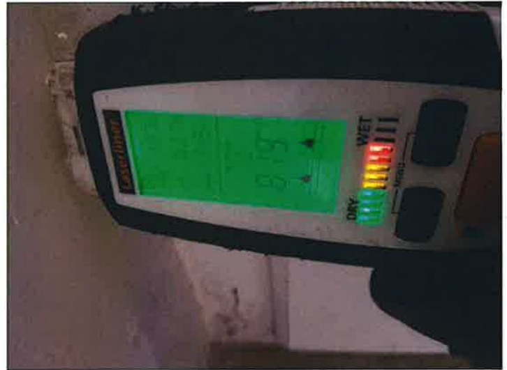
High moisture readings noted to front/ internal walls of property.
