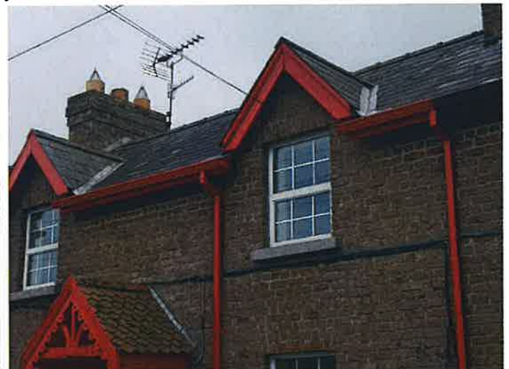
Roof flashings / valleys are prone to leak during strong wind driven rain, monitor. Normal maintenance required.
