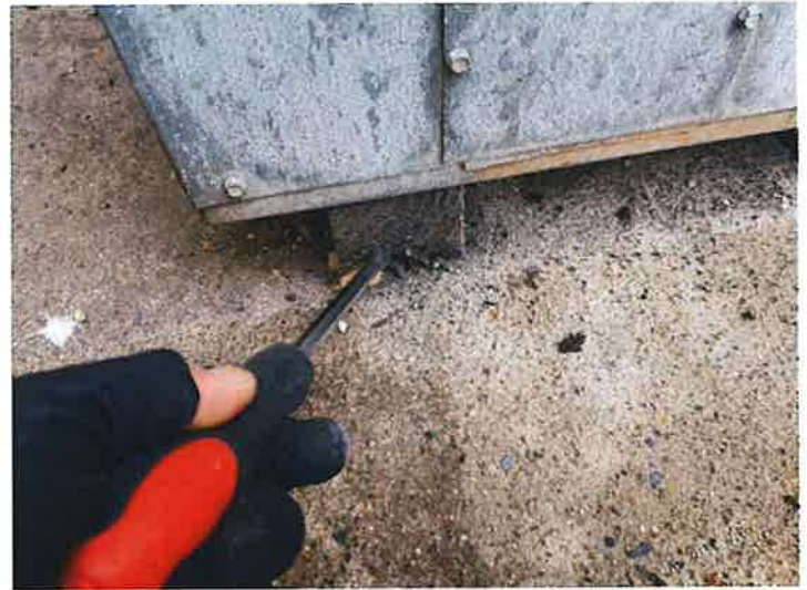
Rotten timbers supporting boiler
