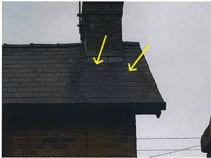
Sample of cracked / damaged roof coverings.
