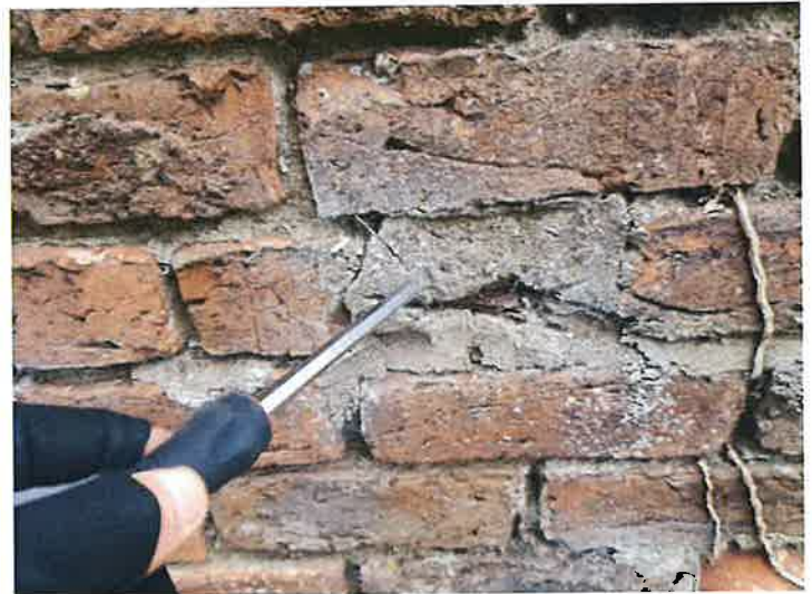
Sections of brickwork walls have been repointed with a cement based mortar, a lime based mortar should have been used.
