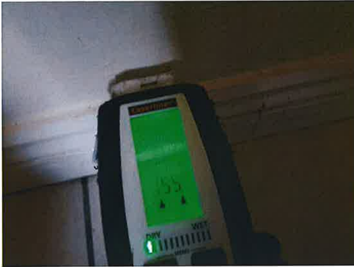
Normal moisture level reading taken at right wall of property.
