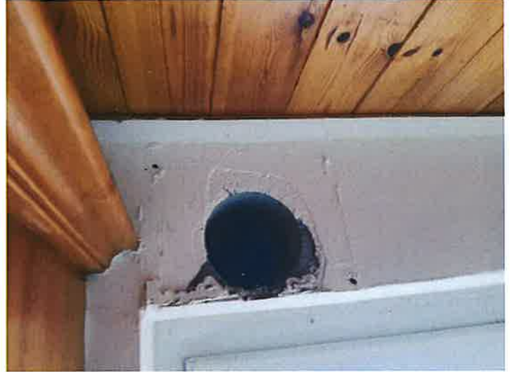
Vent opening partially blocked in kitchen.
