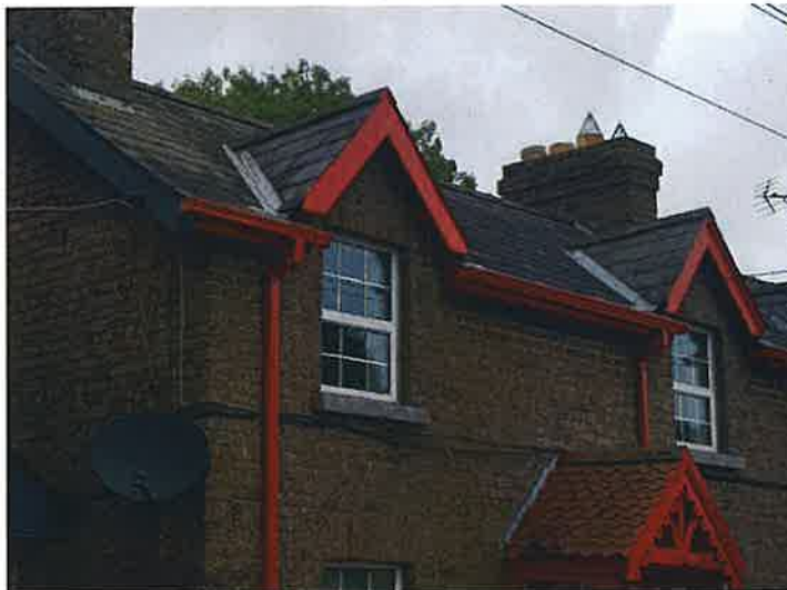
Roof flashings / valleys are prone to leak during strong wind driven rain, monitor. Normal maintenance required.
