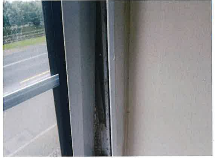
Window hinges require lubrication.
