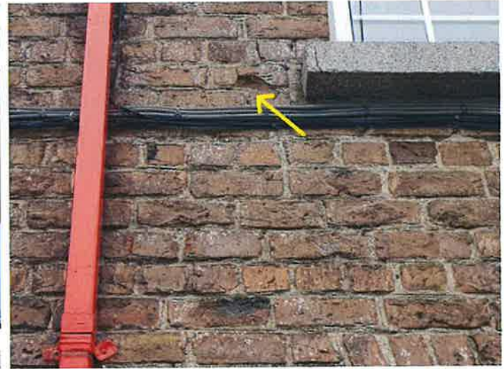
Sample of damaged bricks.
