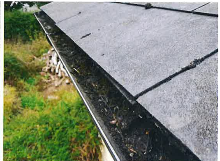
Remove debris from gutters.
