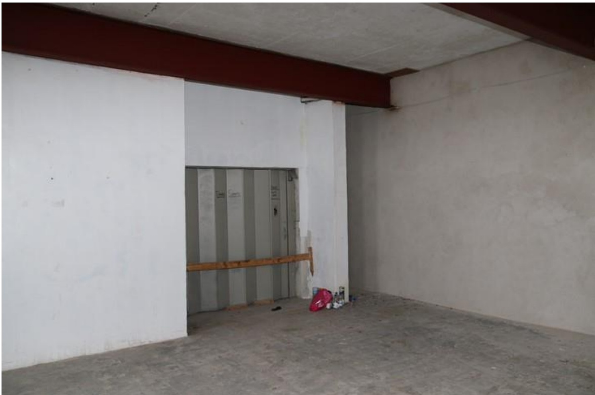
Plate 40: TF-1: Lift in third-floor main room
