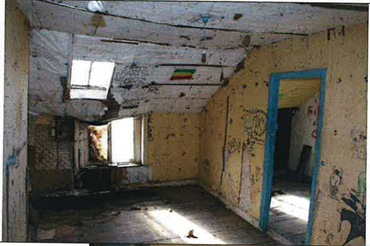
Third (attic floor) front room. No perished roof and derelict state. (5226)
