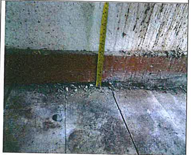
FIGURE 8 SECOND FLOOR PARTITION SAGGED 25MM
