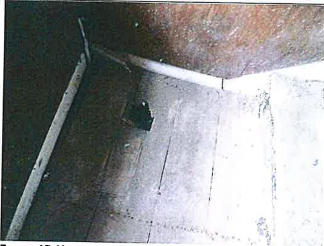
FIGURE 15 HOLE IN STAIRS FIRST FLOOR HALF LANDING
