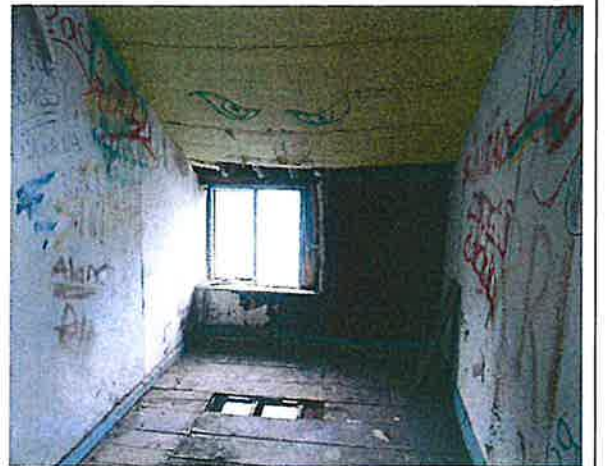
FIGURE 4 THIRD FLOOR ROTTEN RAFTERS AND HEAD
