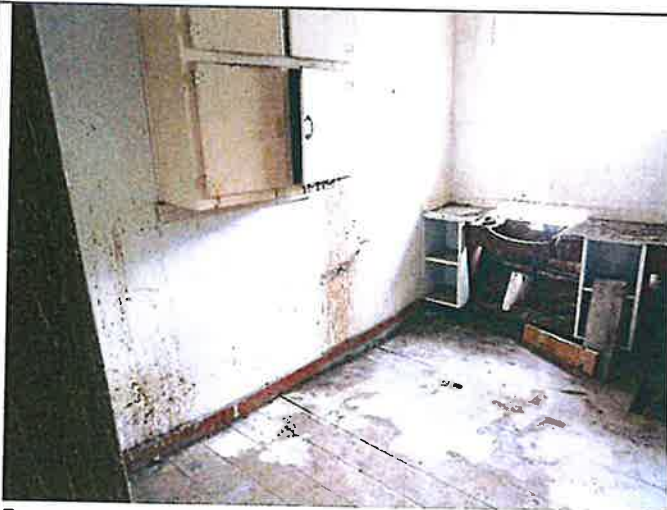
FIGURE 7 SECOND FLOOR PARTITION SAGGED
