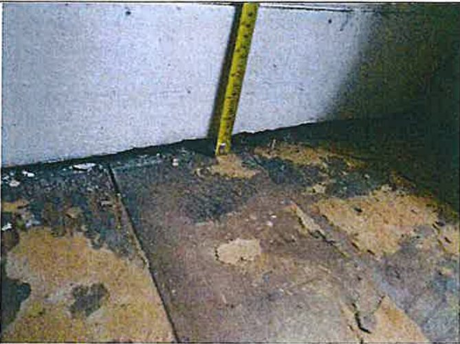
FIGURE 11 FIRST FLOOR PARTITION SAGGED 25MM
