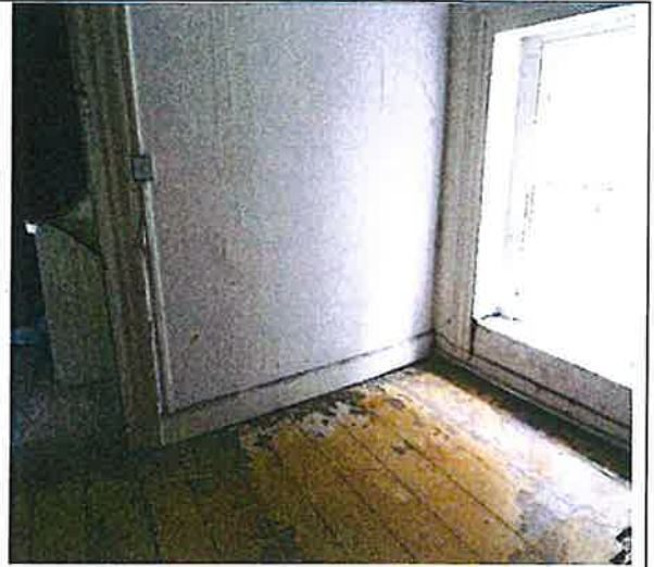
FIGURE 10 FIRST FLOOR PARTITION SAGGED
