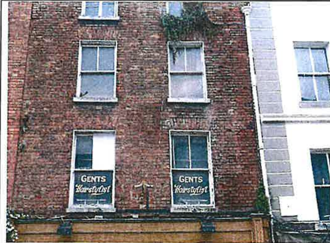
FIGURE 1 FRONT ELEVATION REMOVE VEGETATION AND REPOINT
