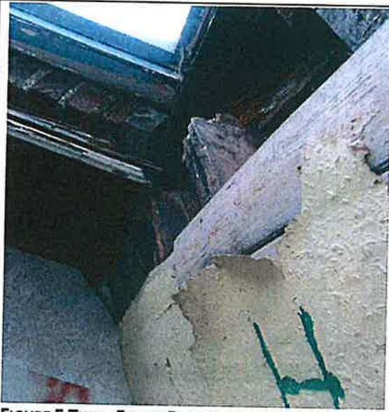
FIGURE 5 THIRD FLOOR ROTTEN RAFTERS AND HEAD
