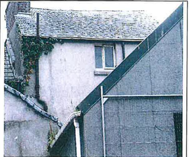
FIGURE 2 REAR ELEVATION SAG IN ROOF
