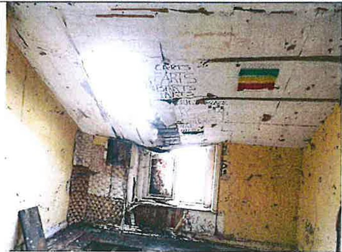
FIGURE 3 THIRD FLOOR ROTTEN RAFTERS AND HEAD
