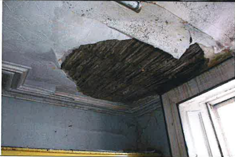
First floor front room ceiling. No plane run corners and perished ceiling. (5242)
