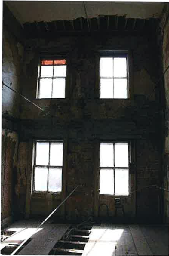
Figure 8: First and second floors and note the second floor is missing.( 3754)
