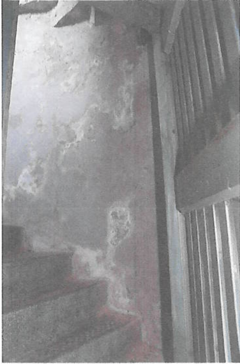
Rain penetration in stairs turret.
