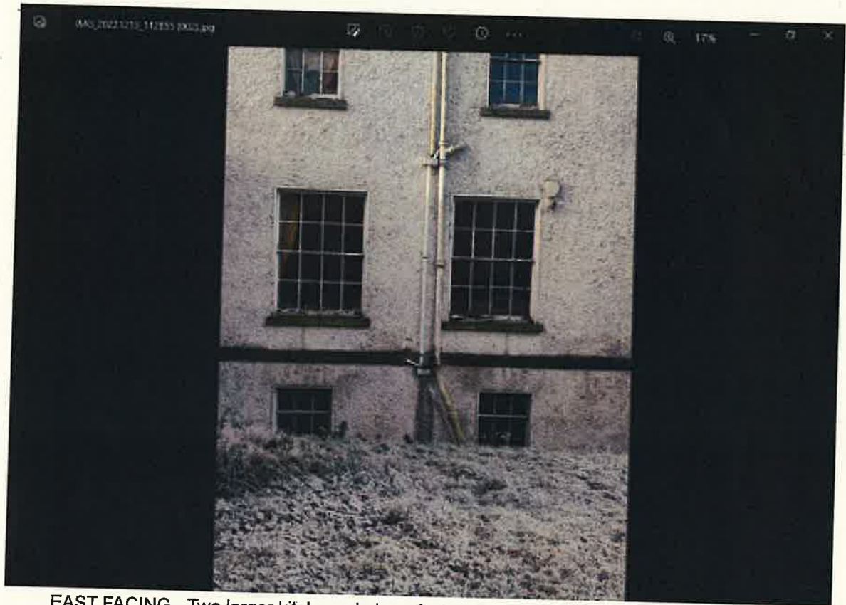
EAST FACING - Two larger kitchen windows facing lawn at side of house (middle of photo)
