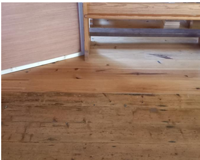
Above: photo of flooring where movement has been detected and flooring around the altar/top of the church area
