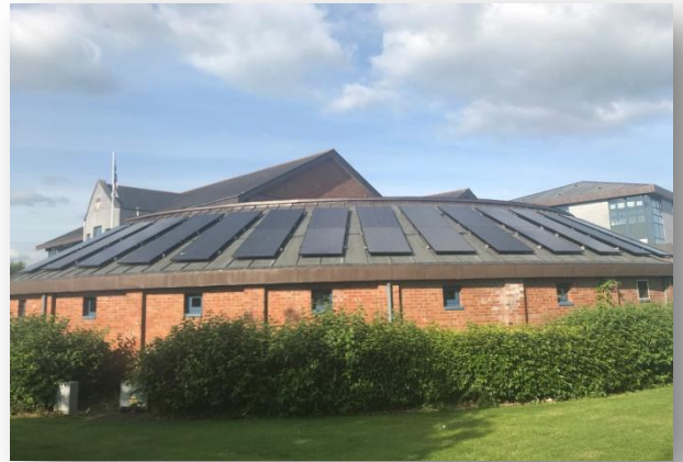
Photograph 7.1 PV panels county hall
