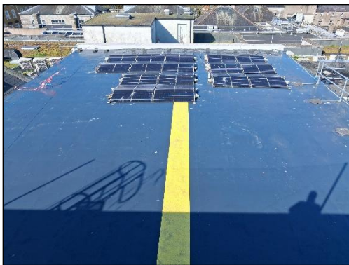
Improvements to the Roof of An Táin Theatre at Dundalk Town Hall
