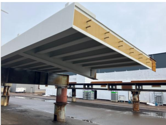
Cantilever footway / cycleway section painted and waiting to be incorporated into deck section one.
