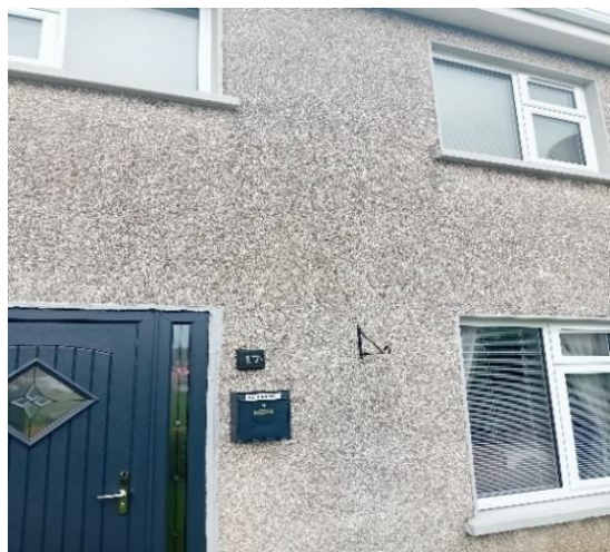
New Windows and Door completed in Dundalk, with funding provided with a HOP
