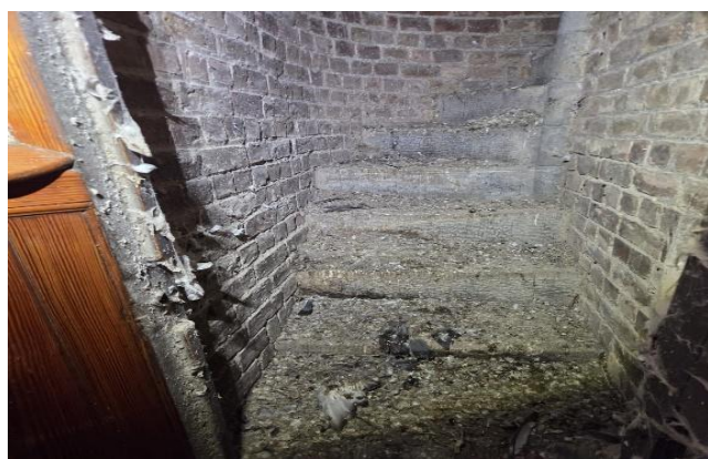
Guano Material on stairwell of Bell Tower
