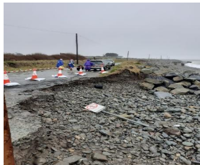
L6218 Storm damage in Salterstown made safe.
