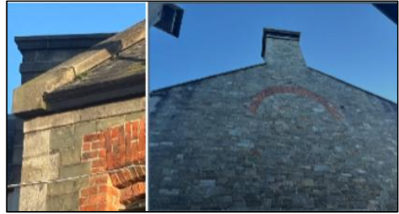
Photos: Existing Stone Walls at County Archives Building in need of Improvement
