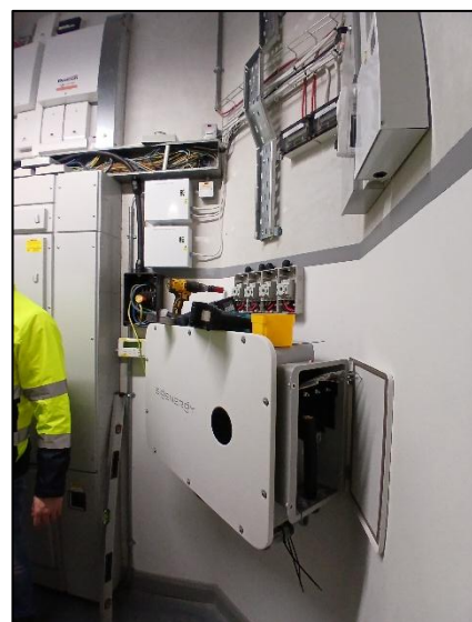
Photo: the new 40kW inverter housed in the L1 Switch Room at the Dundalk Sports Centre
