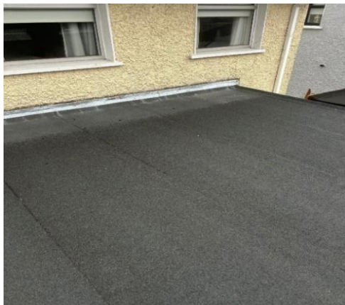
Replacement Flat Roof completed in Drogheda with funding provided with a HOP
