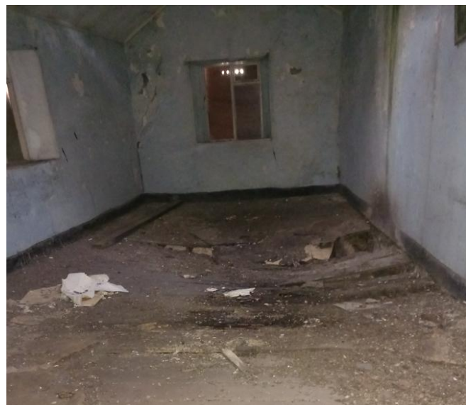
Interior floors subsiding within West Gate House
