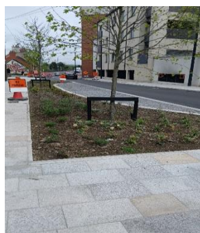
Bridge Street (Phase C) – Overhead cables and ESB Poles removed & Soft Landscaping Complete
