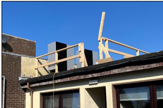
Heat Pump positioned on Dundalk Fire Station's Roof, Surrounded by Temporary Edge Barriers
