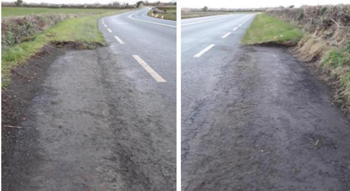
Enhanced hard shoulder Scheme works on the R132 Valley Inn to Dunleer. Re-exposing 1.2m hard shoulder hidden by verge providing greater safety for Pedestrians and Cyclists
