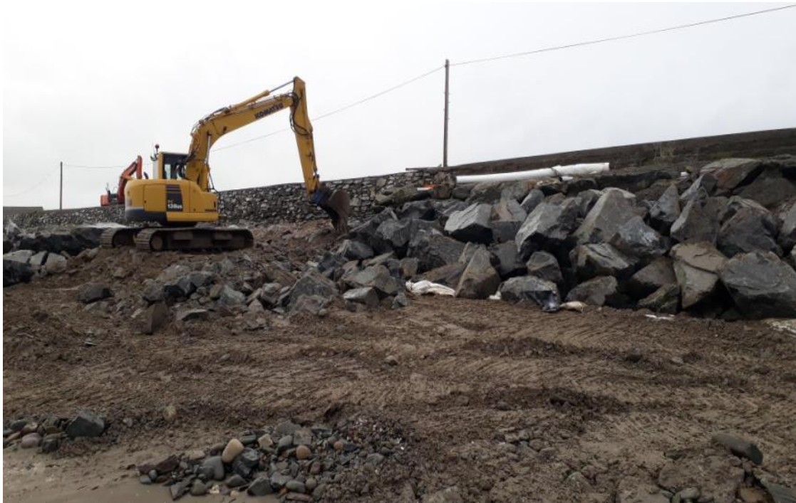
Rock Armour protection to Coast road at Port Beach
