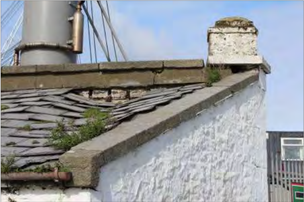
Plate 16: Close-up of outbuilding associated with lighthouse, showing damage to lean-to roof, facing northwest
