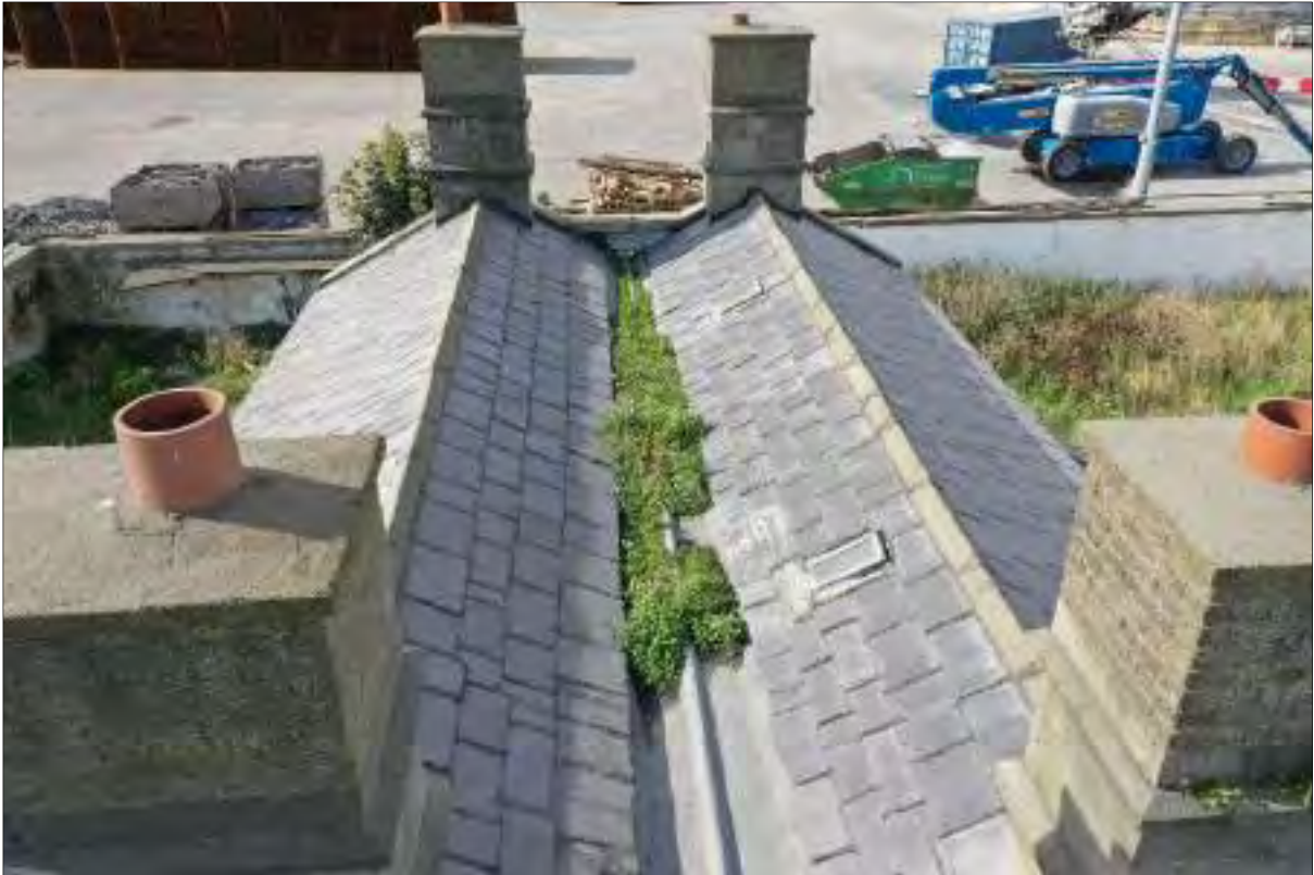
Plate 14: Aerial view of valley to keeper's house, facing southwest – the internal valley is in need of cleaning and unblocking
