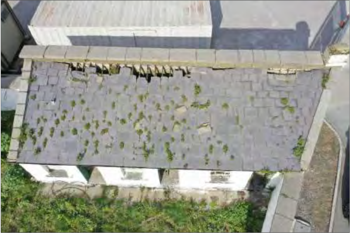
Plate 15: Aerial view of outbuilding associated with lighthouse, showing damage to lean-to roof
