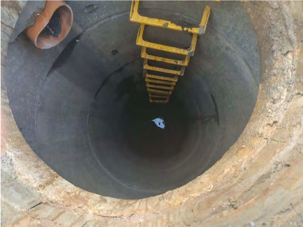
Photograph 4: Surface Water manhole at Location 2.
