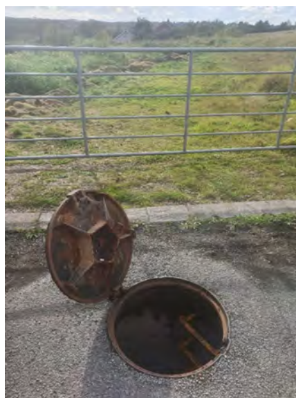
Photograph 1: Surface Water manhole at Location 1 for connection.
