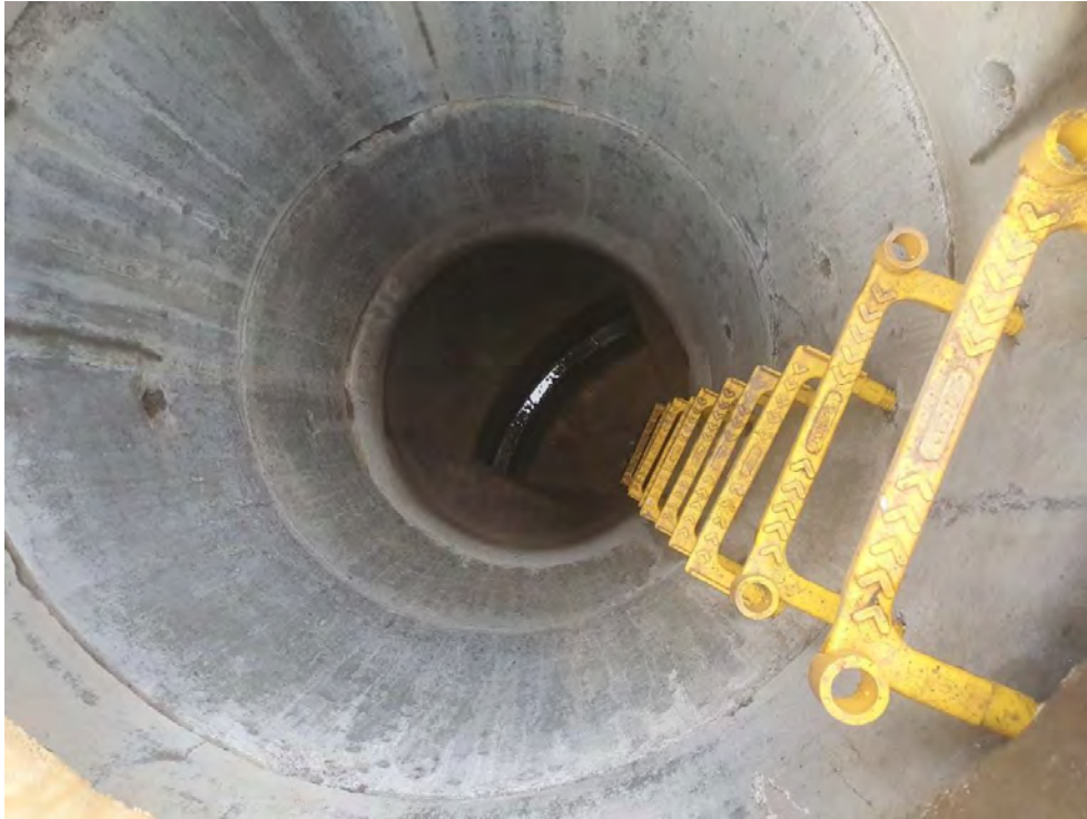
Photograph 2: Surface Water manhole at Location 1.
