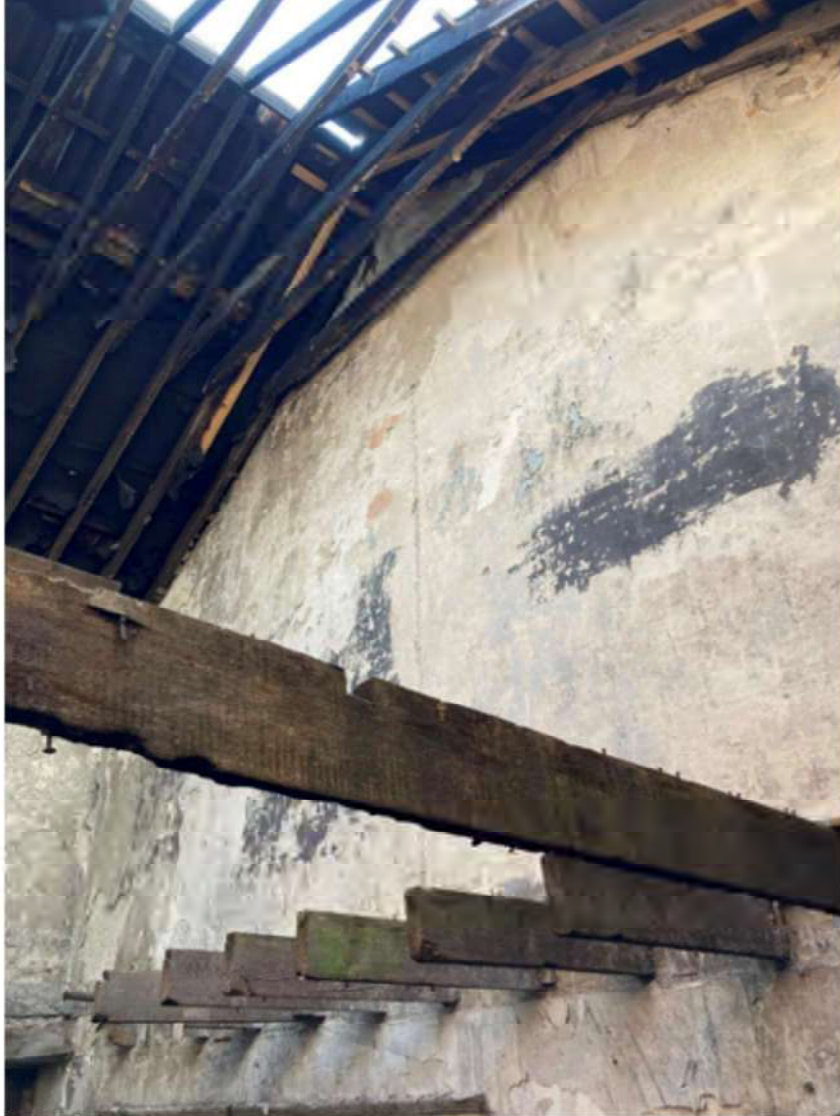
Plate 0.9 View towards ridge showing; charred rafters with collar beams covered to the east with corrugated iron and open to the west; A rafter along the party wall has been sistered and new timber purlins have been laid to provide support to roof cladding of adjacent building.
