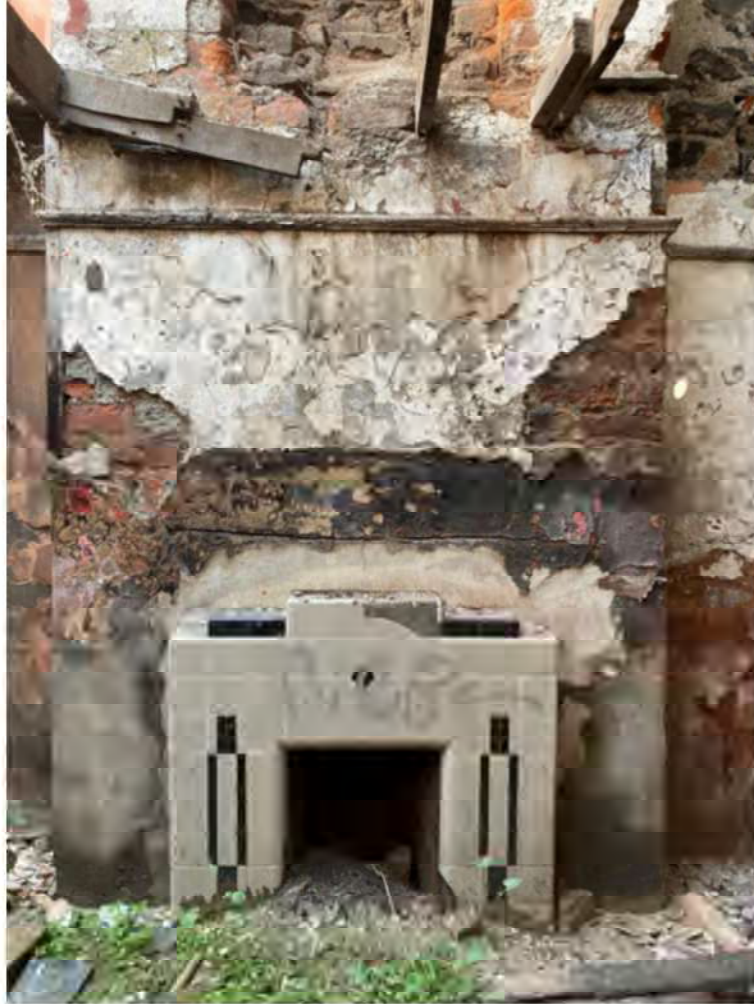
Plate 0.3 North wall showing: the chimney breast with 1950's art deco ceramic tile fire surround; lime render over brickwork at upper level, timber moulded picture rail under collapsed timber first floor structure
