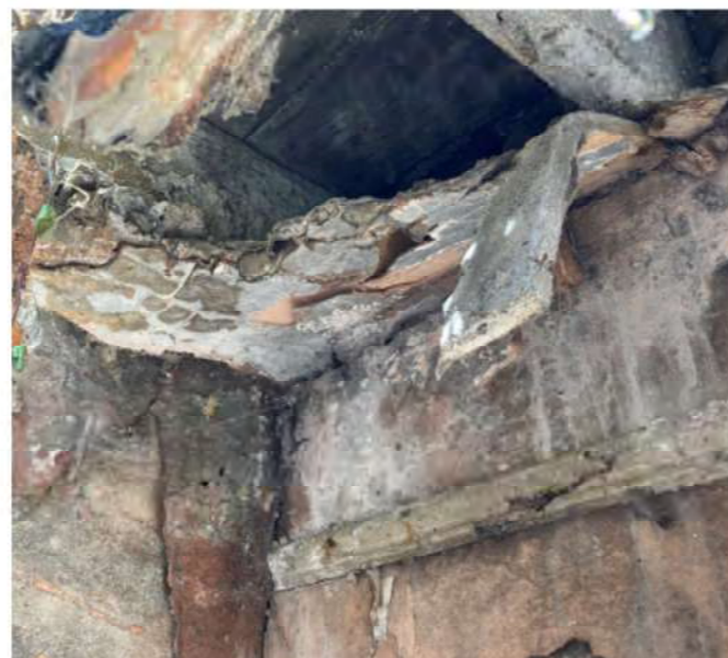
Plate 0.15 View of moulded timber picture rail and remains of later plasterboard ceiling
