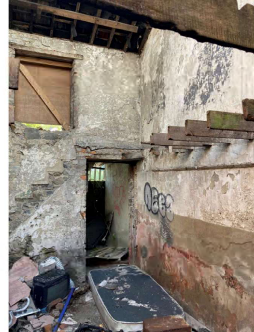
Plate 0.10 View towards ridge showing; charred rafters with collar beams covered to the east with corrugated iron and open to the west; A rafter along the party wall has been sistered and new timber purlins have been laid to provide support to roof cladding of adjacent building.
