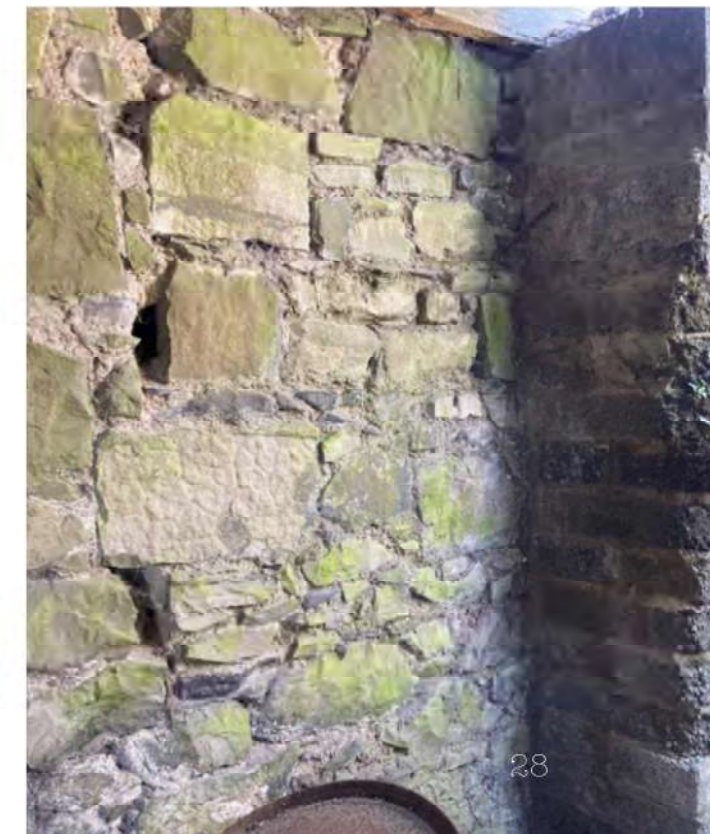
Plate 0.12 View of rear stone wall within covered yard showing the extension of crack to base of wall with large openings within structure
