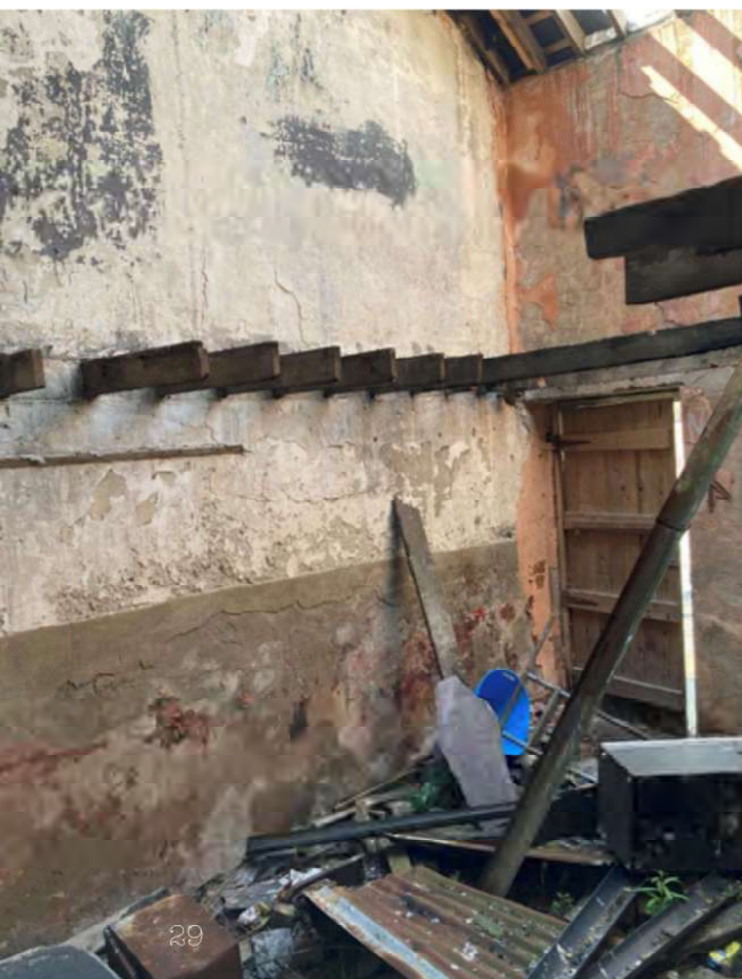
Plate 0.5 South separating wall showing: liquid tanking membrane over lime plaster at lower level; collapsed timber first floor structure; half round cast-iron gutter within rubble.
