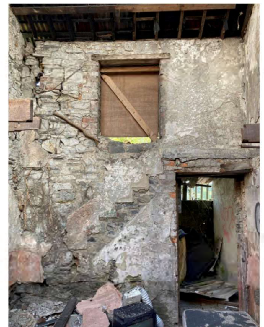
Plate 0.8 View towards east wall showing; significant cracks in north-east corner; root system within wall structure in north-east corner; outline of timber stairs in lime plaster; openings formed in red brick; timber heads to door and window; gypsum plaster at lower level to north wall and lime plaster to rear wall; windows and doors are lost.
