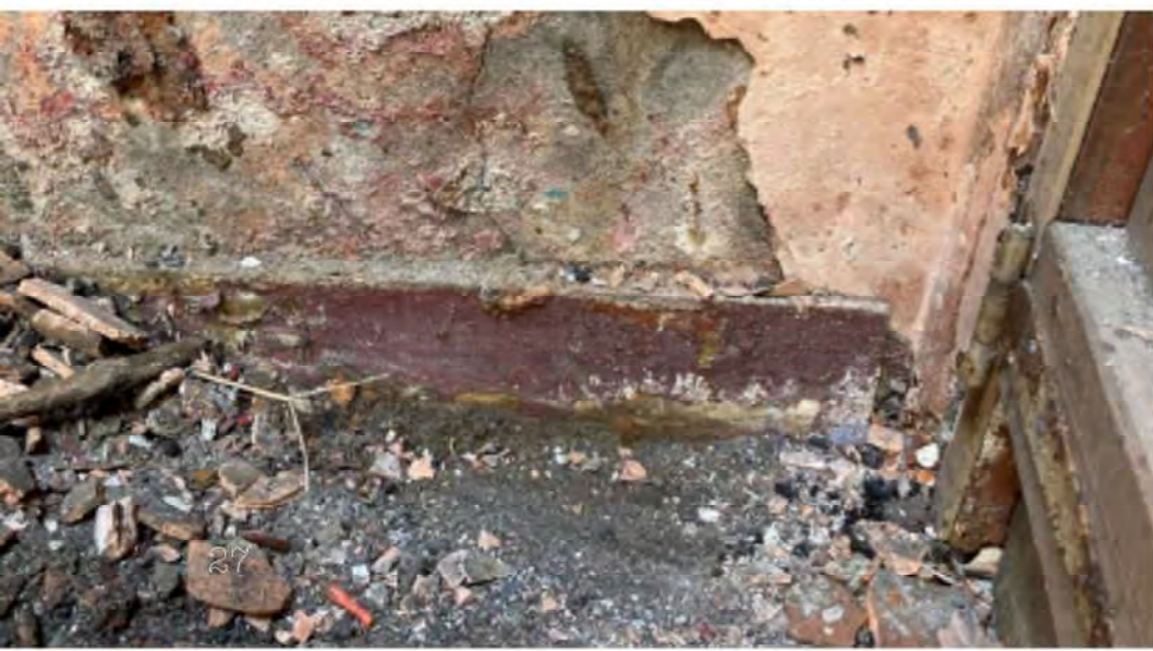
Plate 0.15 View of timber skirting adjacent entrance door
