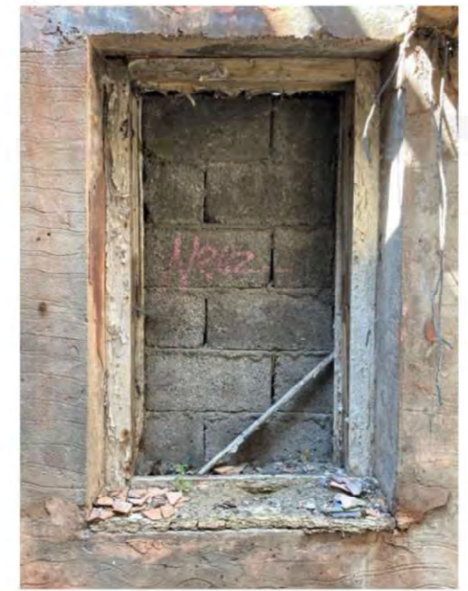
Plate 0.14 View of ground floor boxed sash frame to front wall
