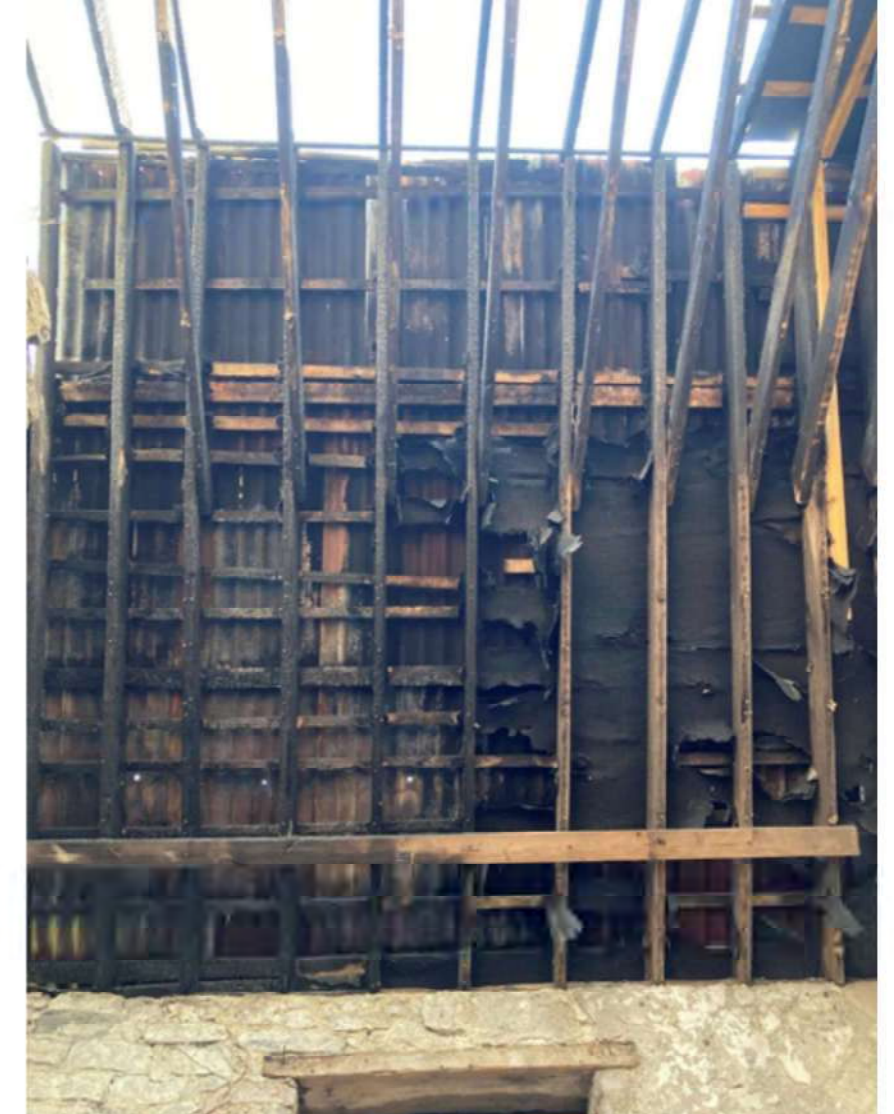
Plate 0.7 View towards east slope of roof showing; charred timber trusses with collared beams; charred timber purlins and felt with corrugated sheeting over; timber head to first floor window.
