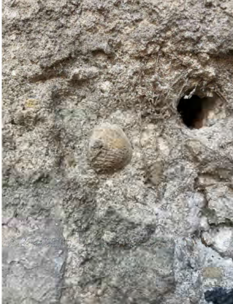
Plate 0.15 View of local sea shells forming part of the aggregate within the original lime plaster
