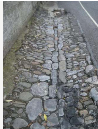
Fig. 5. 24: Cobble drain, Millmount
