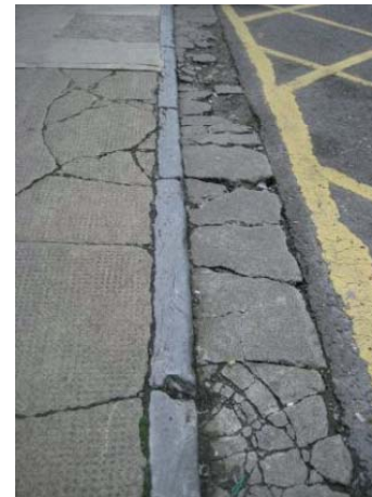
Figs 6.64 to 6.75 (top left to bottom right): Historic paving elements - kerbs, drains paving To be retained as part of public realm enhancement schemes
